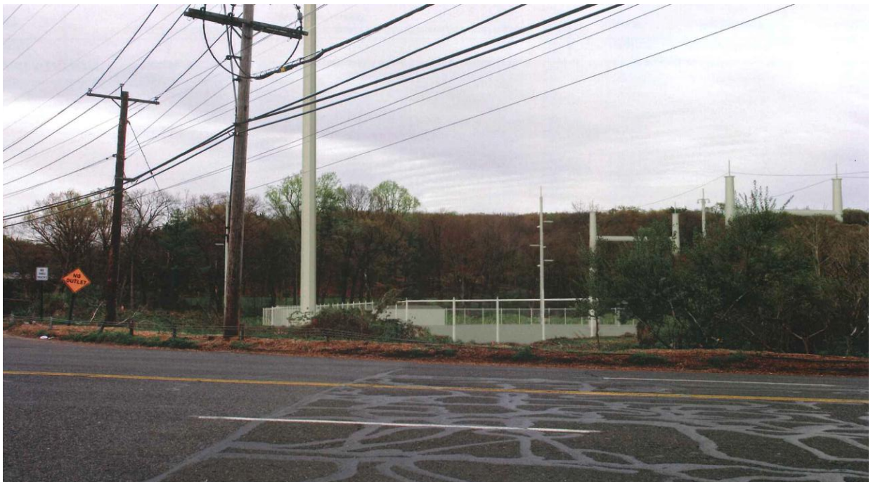
Figure 3 B: Photostimulation of substation from Old Stratford Road, west of Route 8 south exit ramp. (UI 7)
