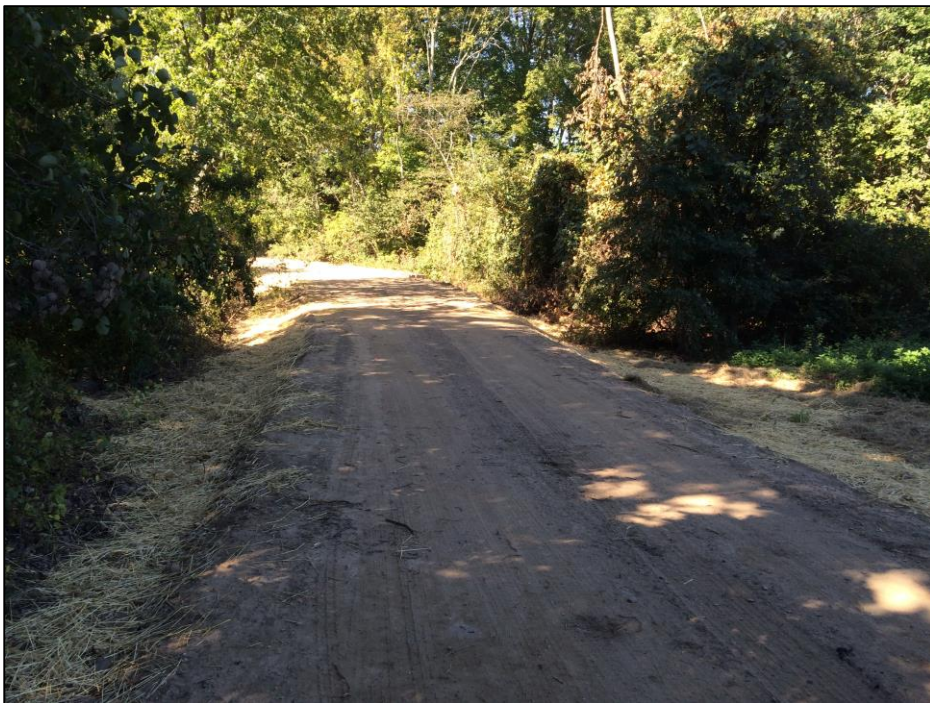
Photo #8: All bare areas around the Day Street culvert seeded and temporarily stabilized with straw. (9/24)
