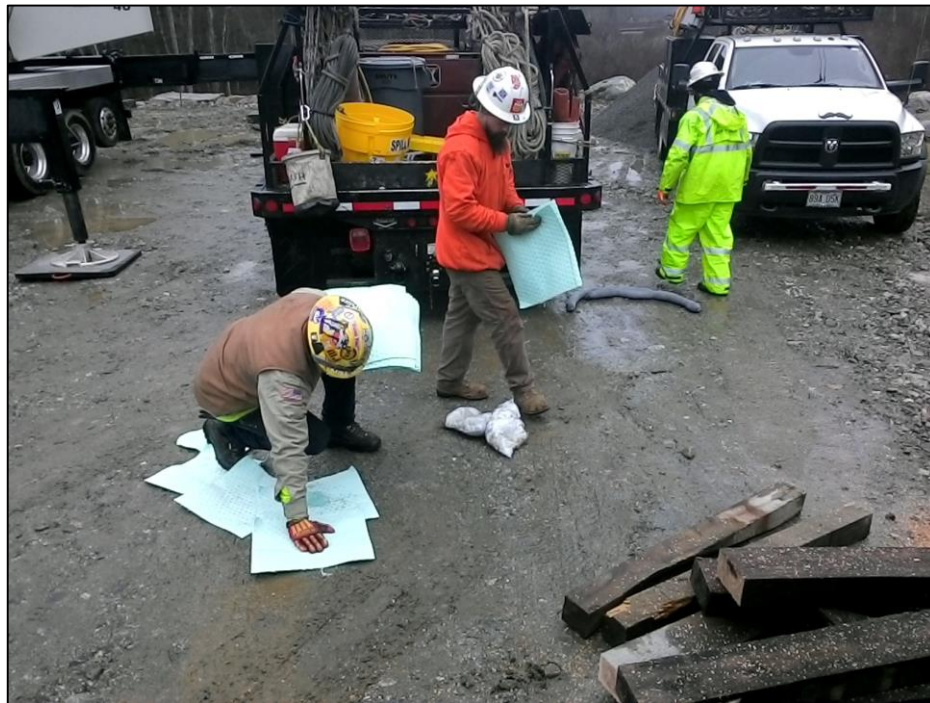
Photo #6: Crew immediately contained and cleaned up the area.
