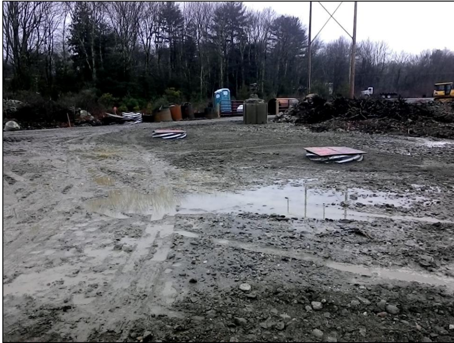
Photo #11: Evidence of muddy access roads.
