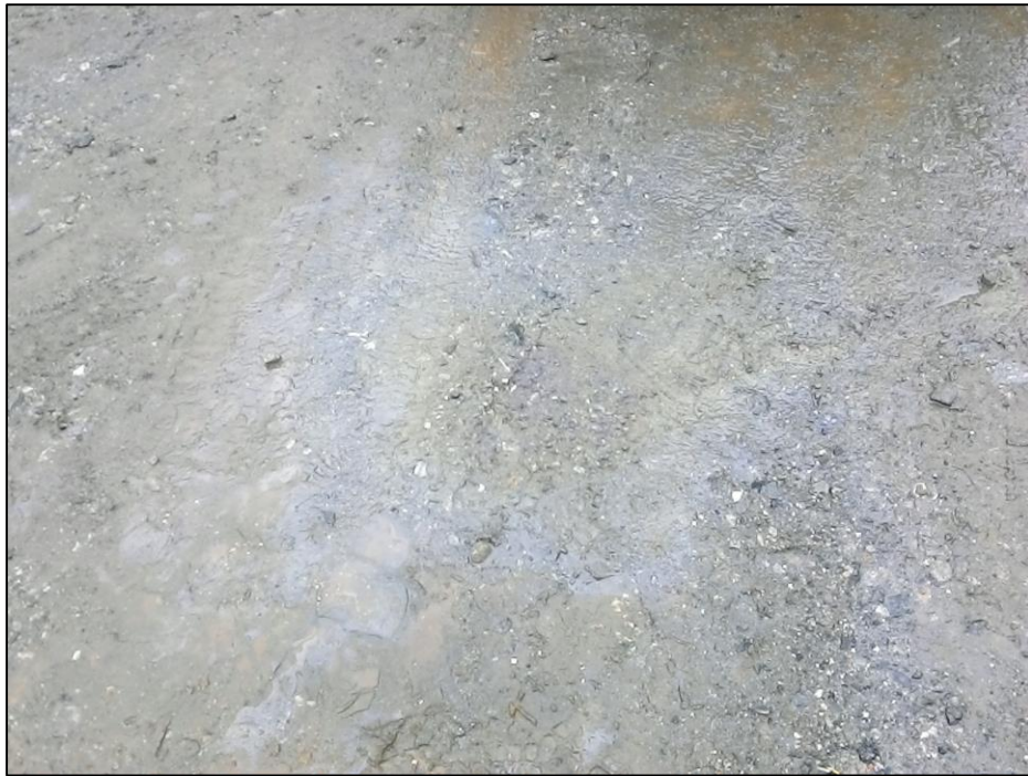
Photo #5: Observed Petroleum based spill on pad 160.
