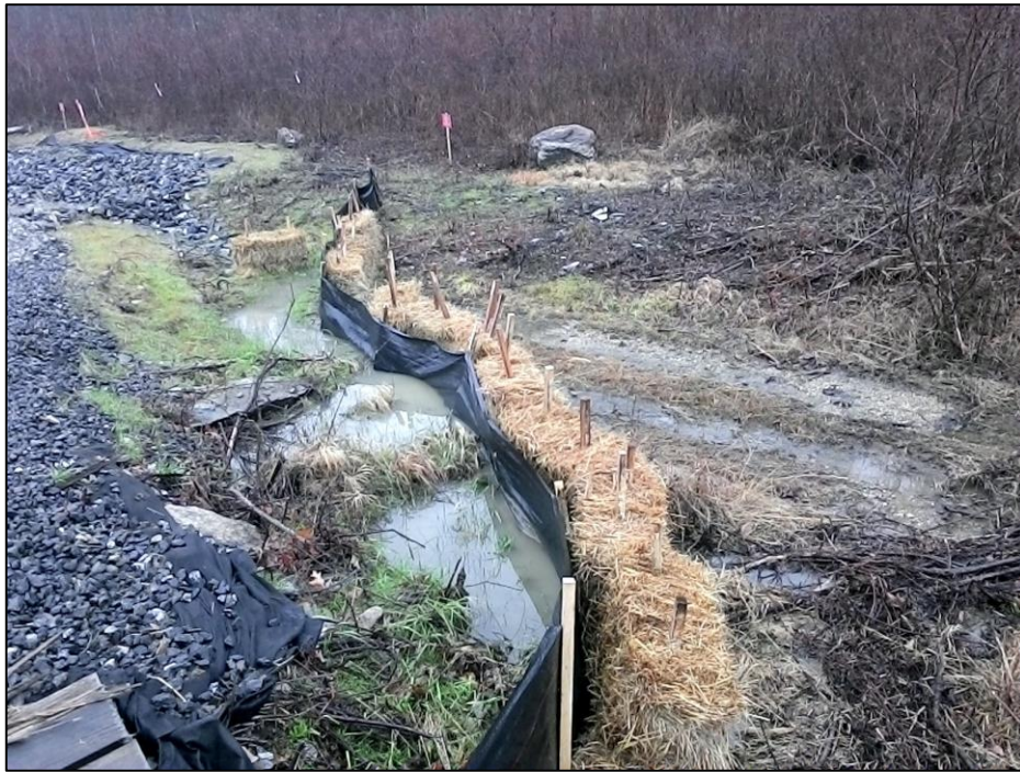
Photo #3: Straw bale reinforced silt fence at discharge point downtime of Str 157.
