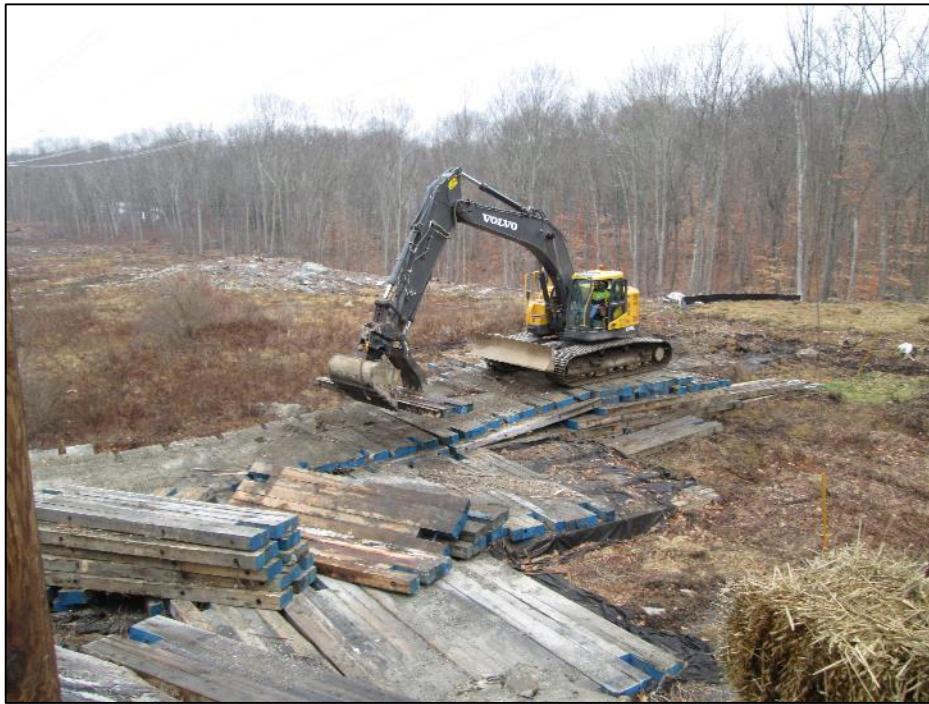
Photo #7: Removal of wetland mats and restoring to pre-construction grades and slopes at Str 104. (12/16)
