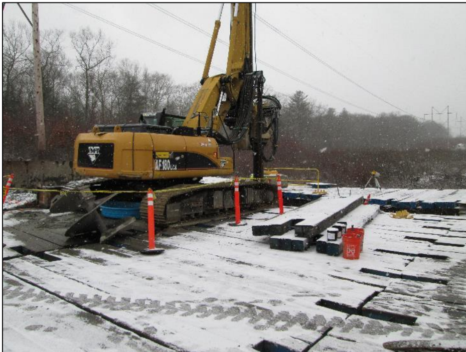
Photo #8: Observed child pool under drilling machinery for precautionary measures at Str 161. (12/11)
