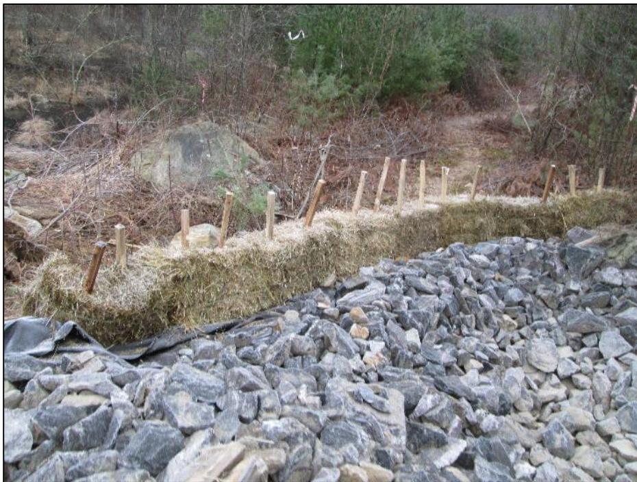
Photo #4: Observed hay bales re-installed correctly on edge of plunge pool up-line of Str 315. (12/16)
