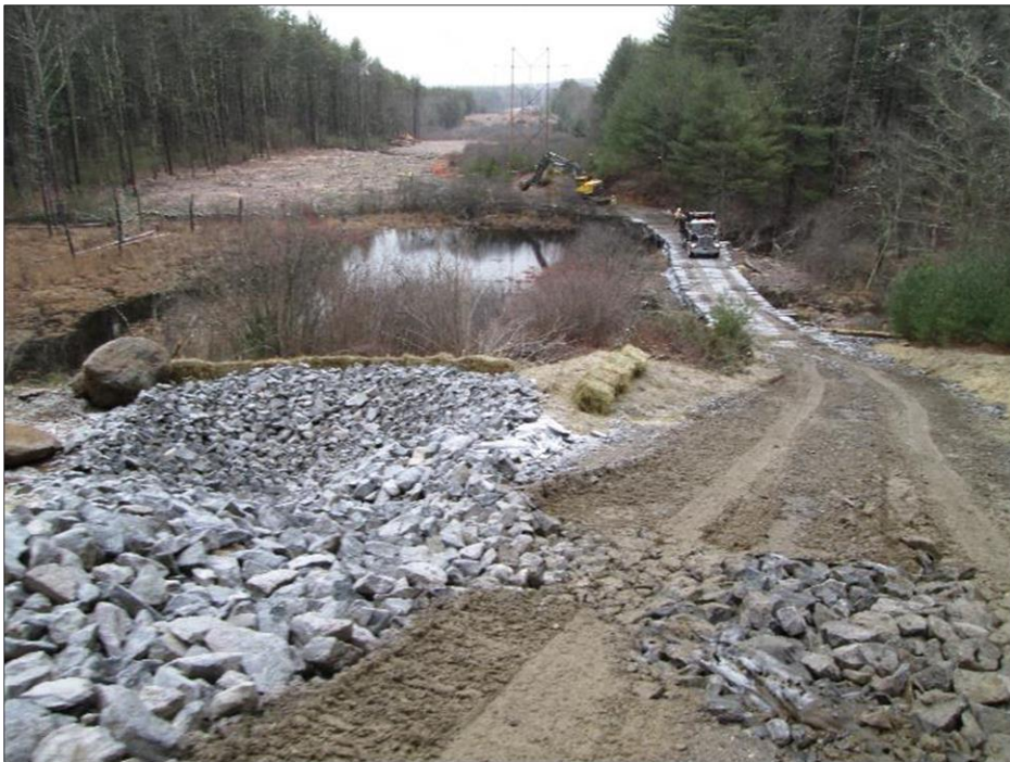
Photo #2: Observed plunge pool, armored water bar and hay bale reinforced silt fence up-line of Str 315. (12/11)
