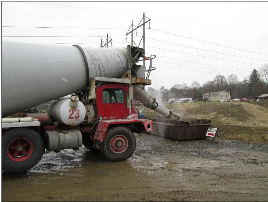
Photo #5: Observed concrete wash-out upland at Str 243. (12/11)
