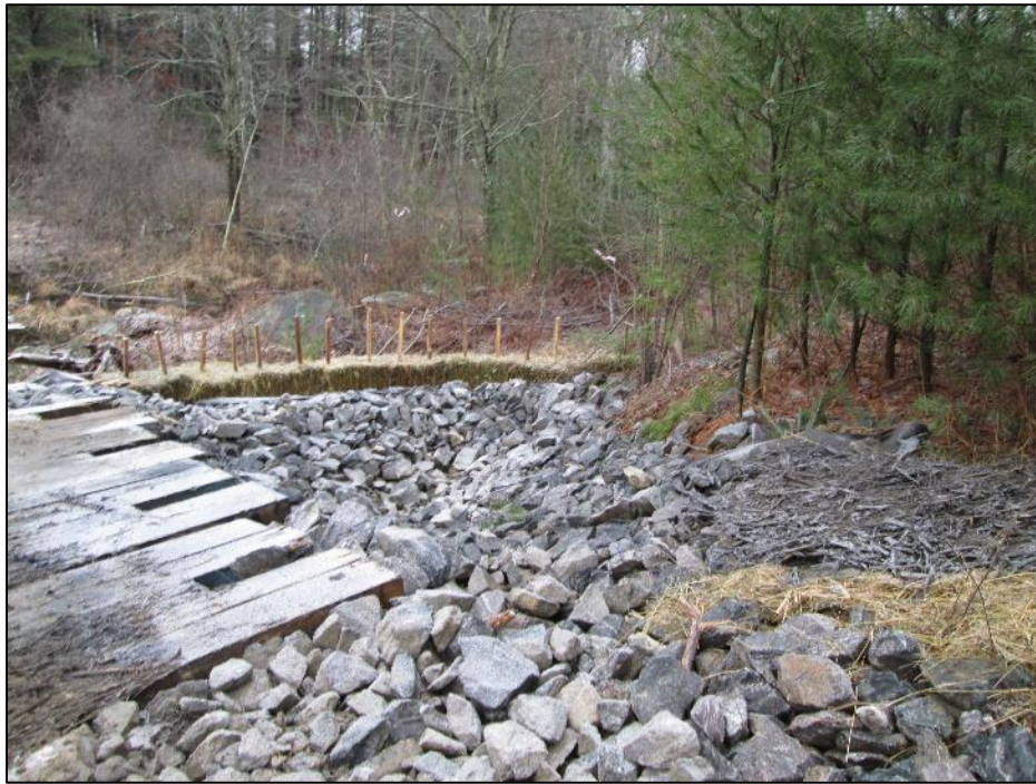
Photo #3: Observed hay bales installed incorrectly on edge of plunge pool up-line of Str 315. (12/11)
