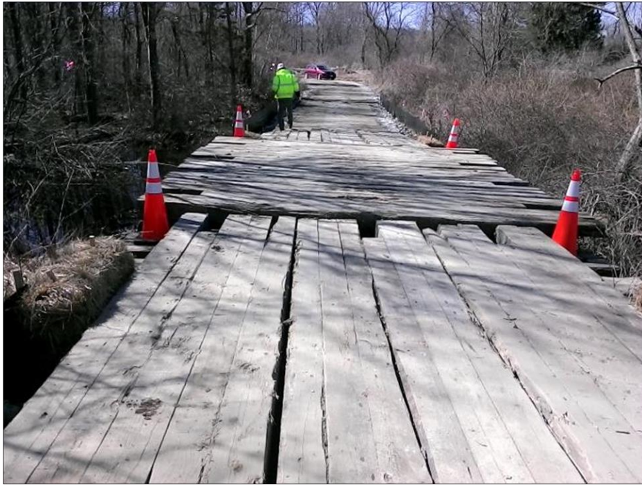
Photo #5: (South of ROW on access from Card Street) View of temporary wetland crossing.
