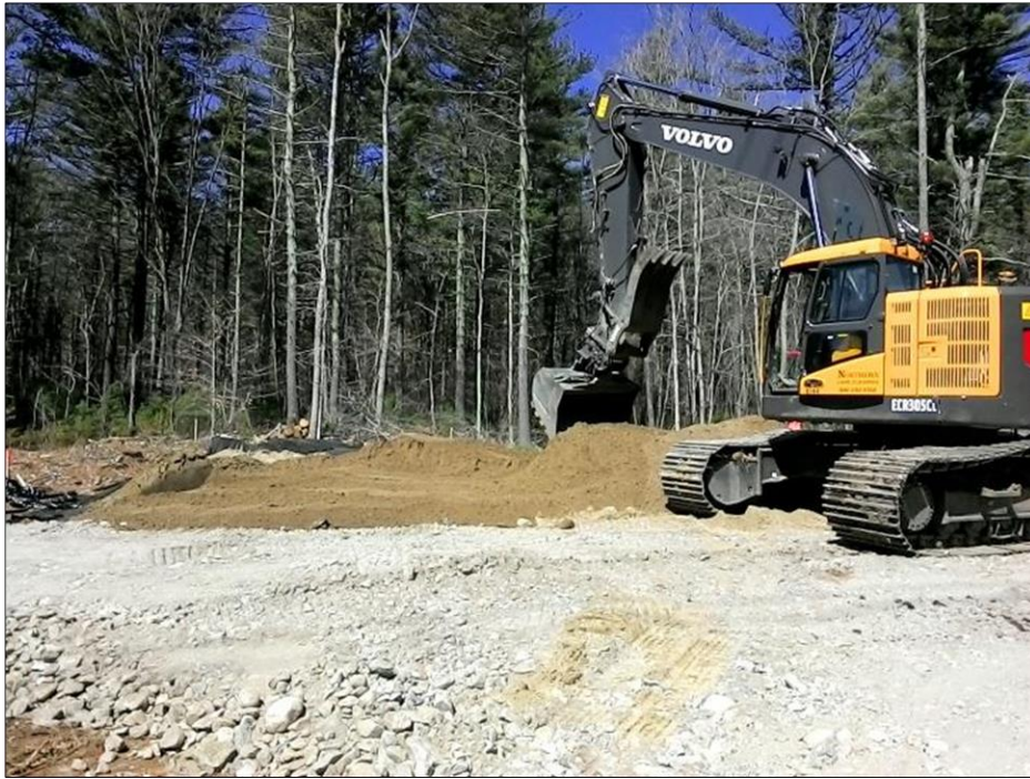
Photo #9: View of installation of filter fabric and buffer sand at pad 85 over area of cultural significance.
