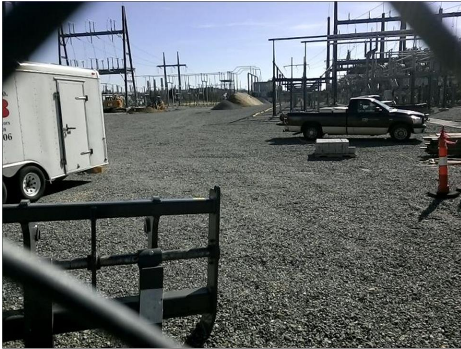
Photo #15: View facing down-line into KS of excavation activities. Straw wattles installed at edge of excavation visible at back center of photo.
