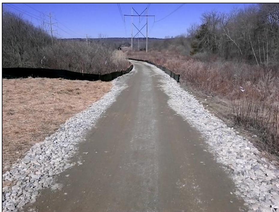
Photo #2: View (up-line toward str 3) of fine material along the top surface of the access road.
