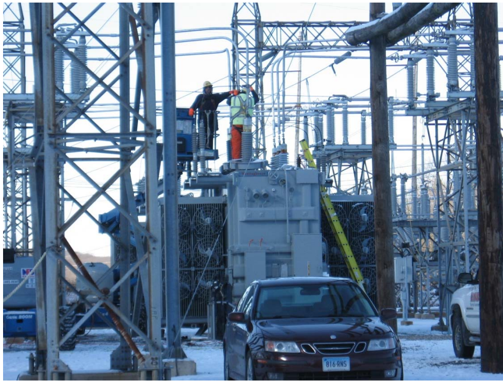
Photo #7: View (facing northwest) of contractors working on aerial bus-way on north side of substation. (not project related)
