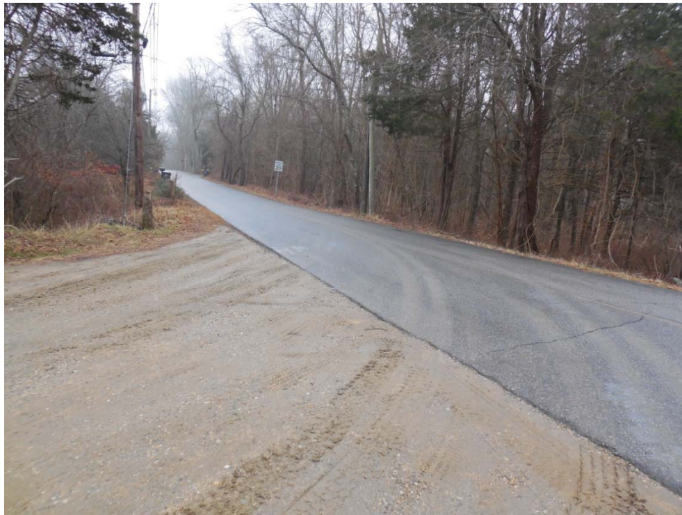
Photo #6: View (facing east) of Card Street, free of significant sediment from access.
