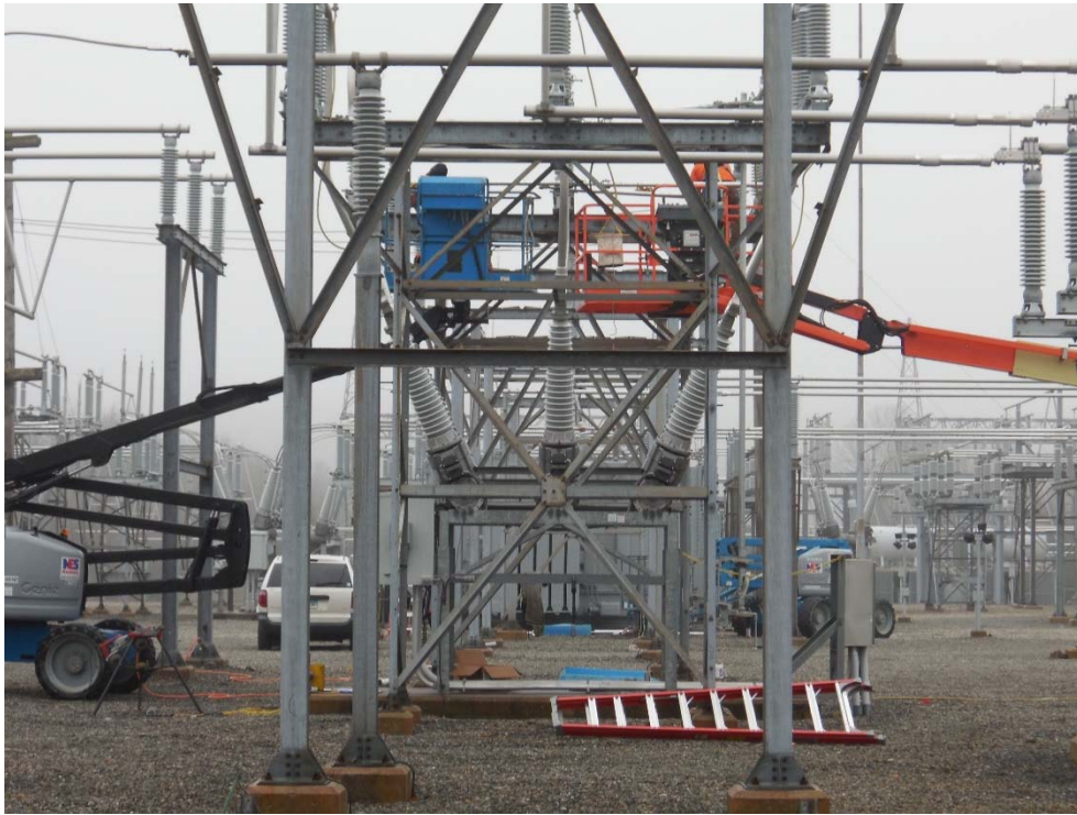
Photo #7: View (facing south) of electrical contractors working on aerial bus-way on north side of substation.
