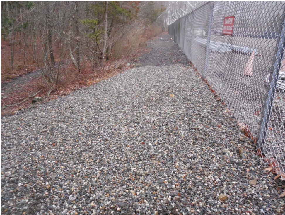
Photo #2: View (facing west) of third (main) runoff outlet at southwestern edge of substation with no apparent sedimentation.
