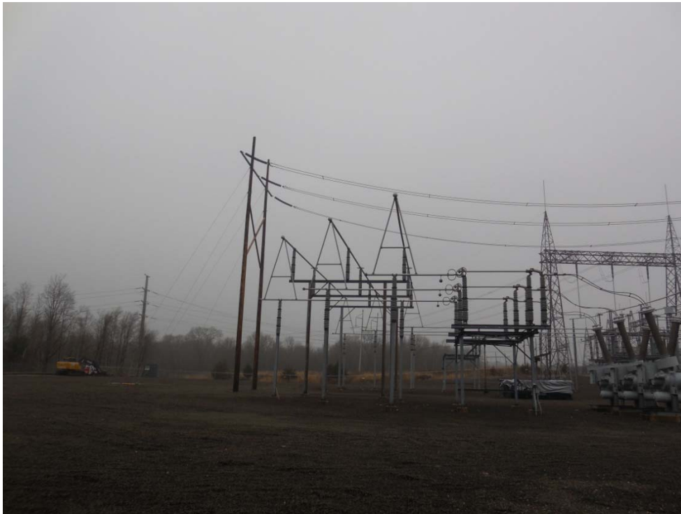
Photo #4: View (facing northwest) of second of two new Wood Pole H-frame Structures.
