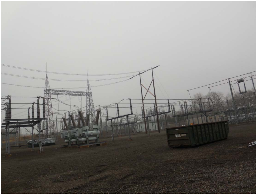
Photo #3: View (facing northeast) of first of two new Wood Pole H-frame Structures and contained, covered stockpile dumpster (left background of photo).
