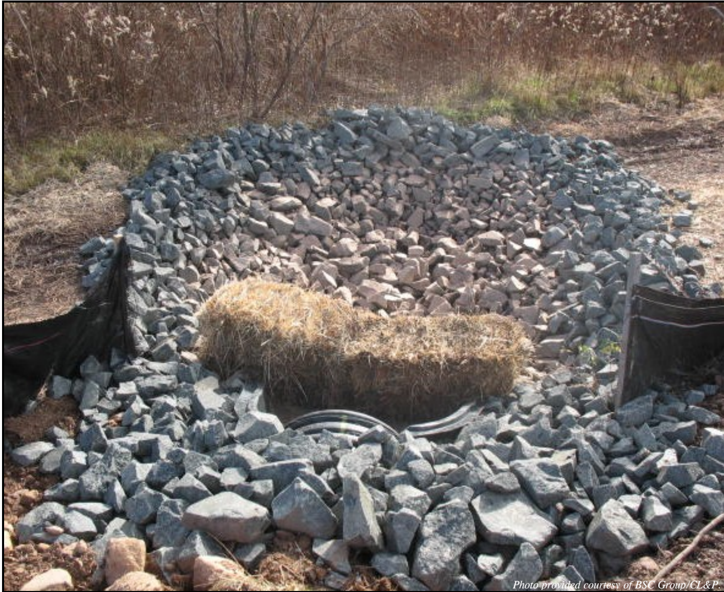
Photograph 7-1 Riprap at outlet of permanent culvert (haybale checkdam in place during construction activities only).
