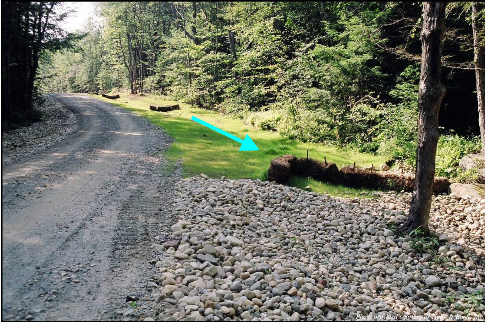
Photograph 4-8 Grass-lined swale underlain with erosion control blanket and containing hay-bale check dams; used to quickly stabilize soils along a construction access road subjected to significant stormwater runoff. Blue arrow indicates direction of flow.
