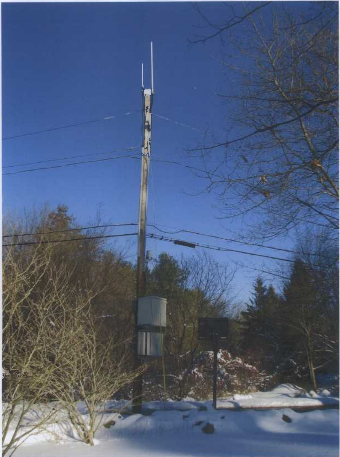
Figure 1: Typical DAS Node 1
