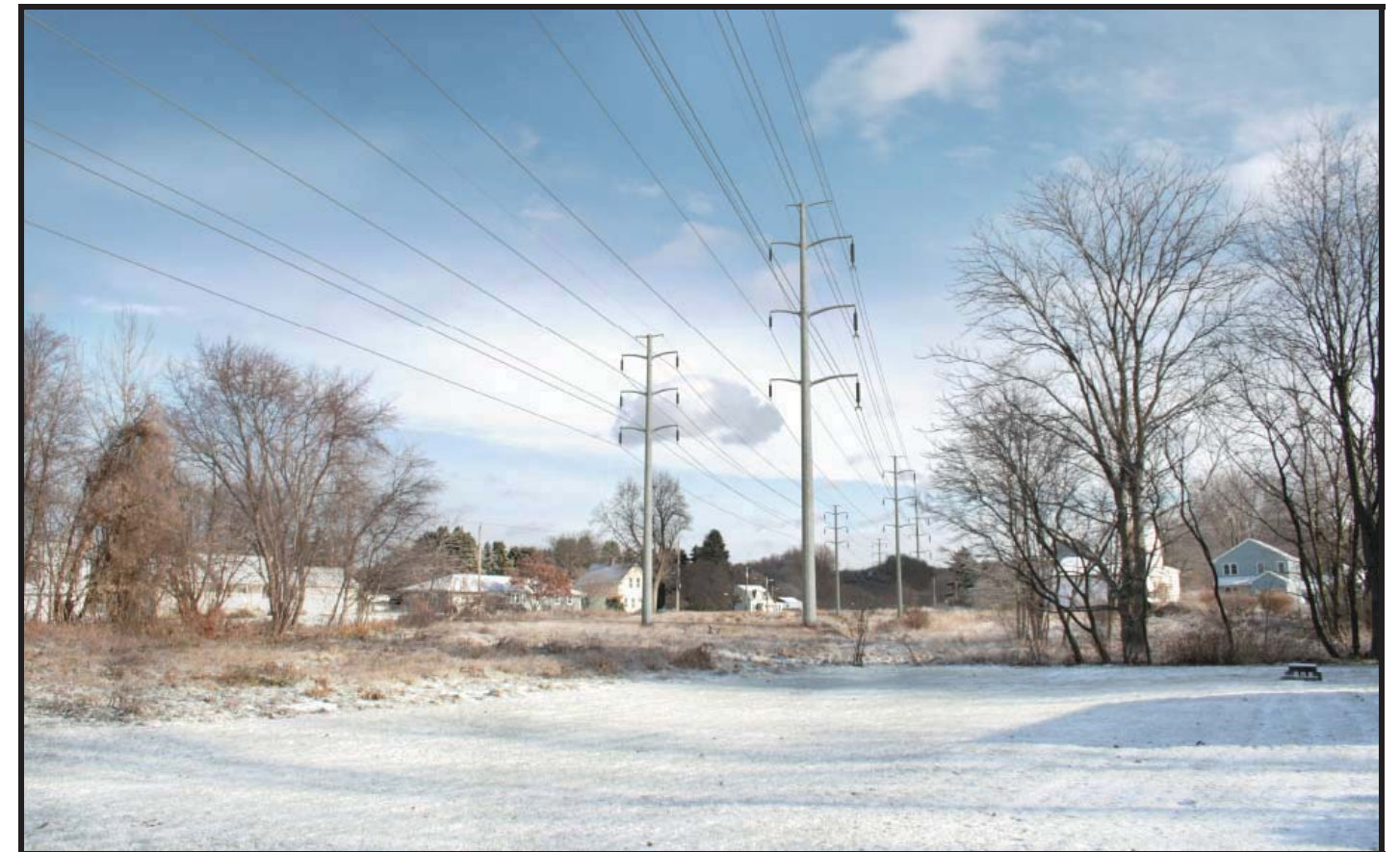
Proposed electric transmission line structures looking north from Wayfield Avenue, northeast of Piper Substation.
