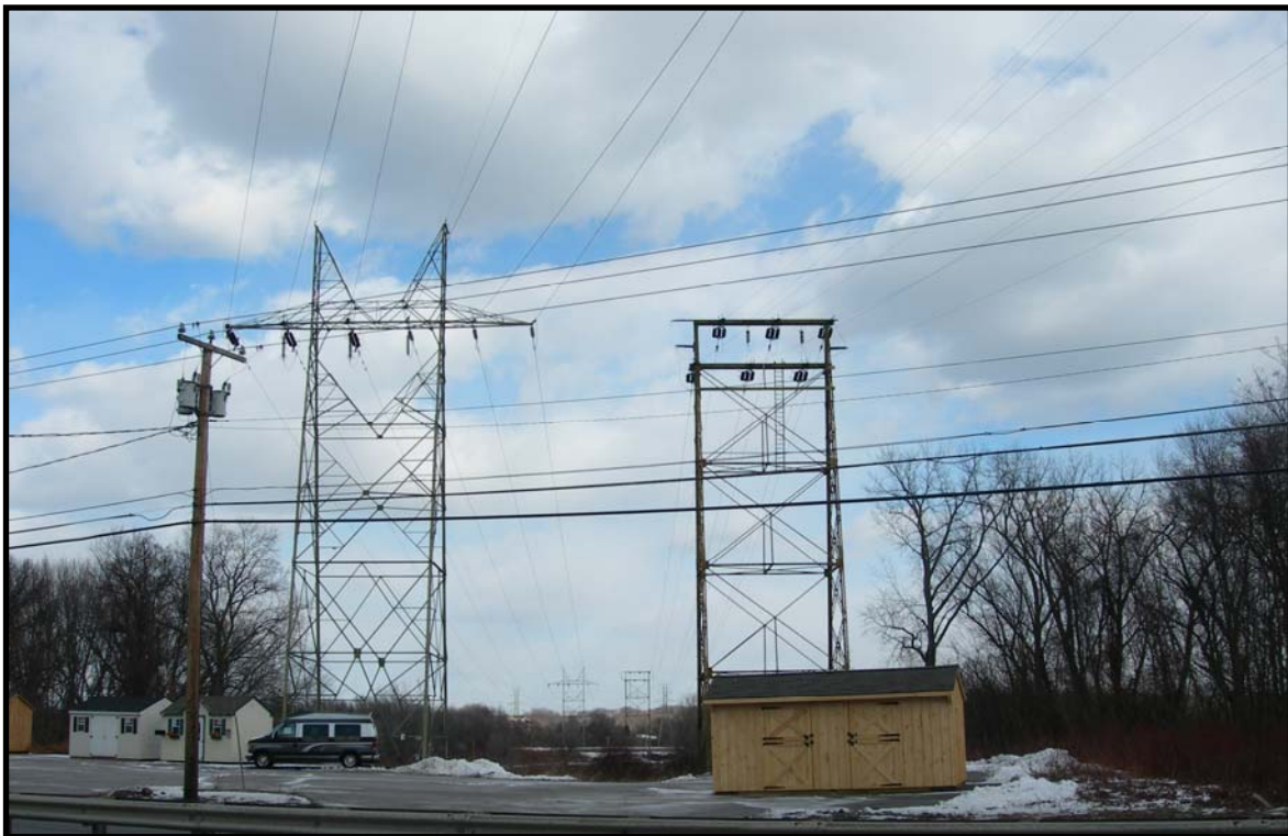
Photo 345-kV Line Route OH-10: View east from Riverdale Street in the Town of West Springfield, MA. This is the crossing location of the Connecticut River.
