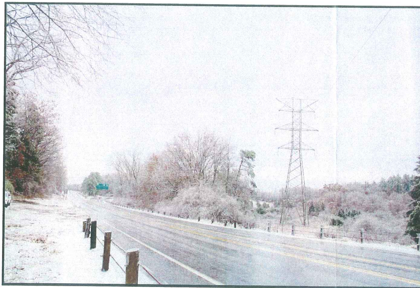
Existing electric transmission line structures looking southwest from State Highway 189, north of North Bloomfield Substation.
