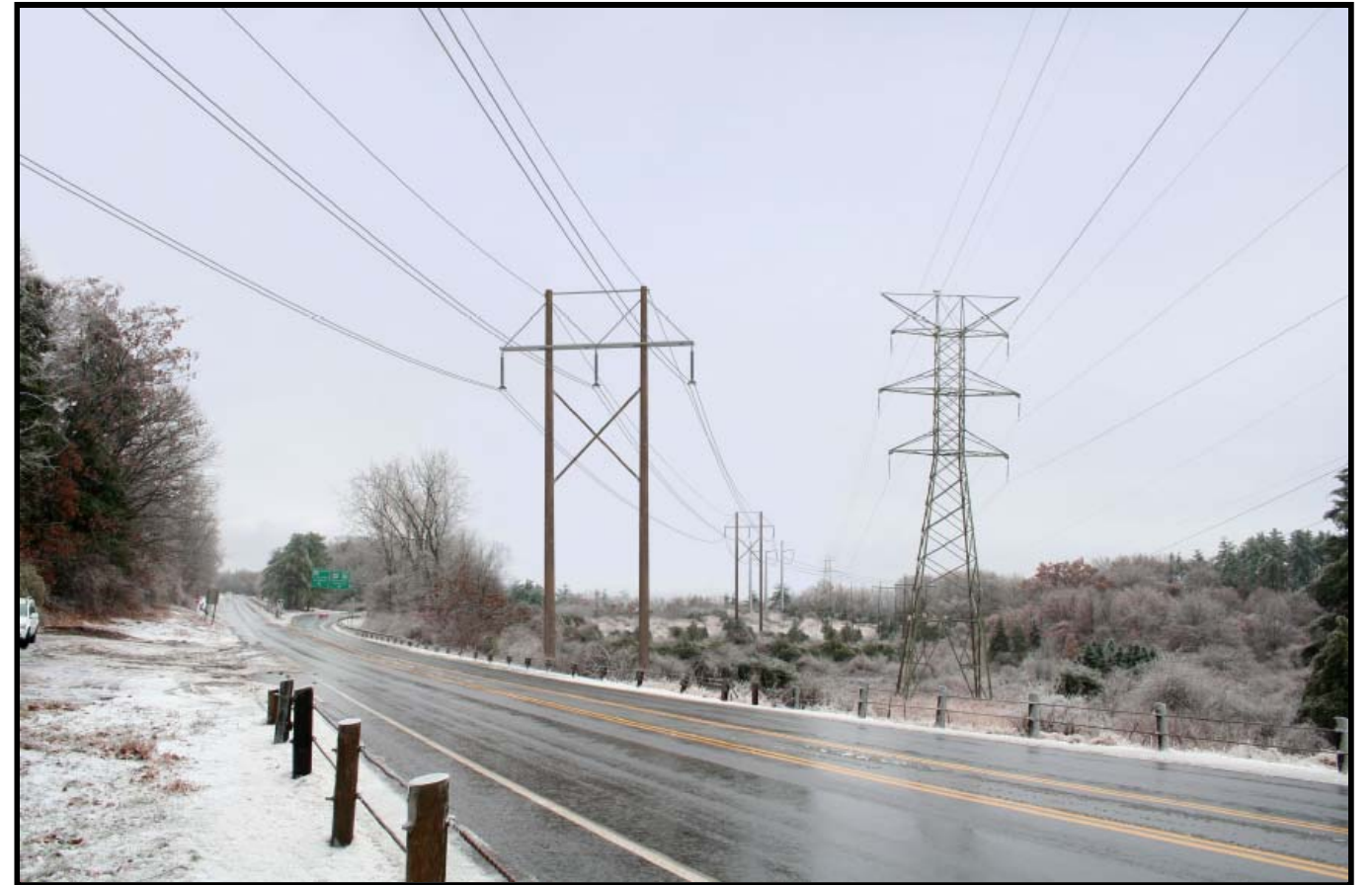
Proposed electric transmission line structures looking southwest from State Highway 189, north of North Bloomfield Substation.
