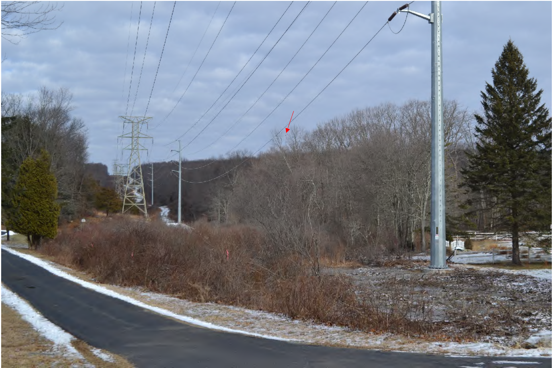
Photograph 4: Prokop Transmission ROW
