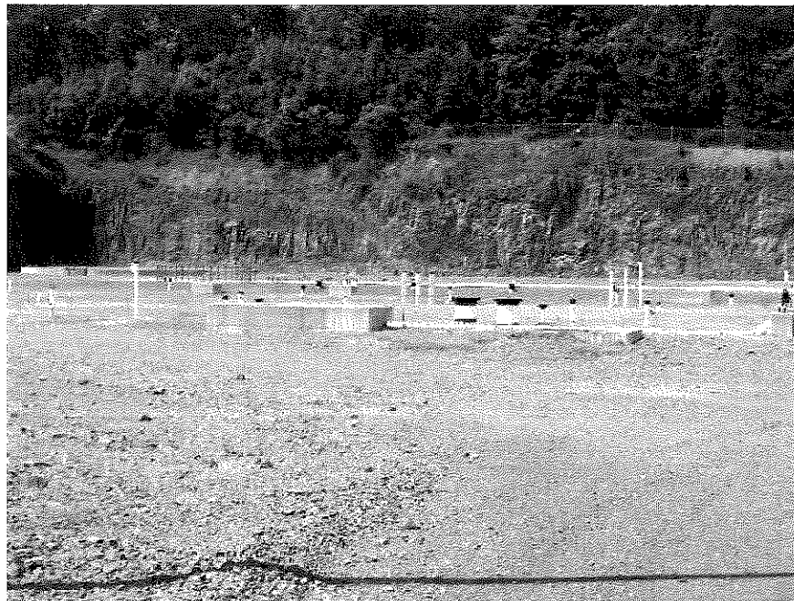
Piping and support for equipment that was removed on west side of main building
