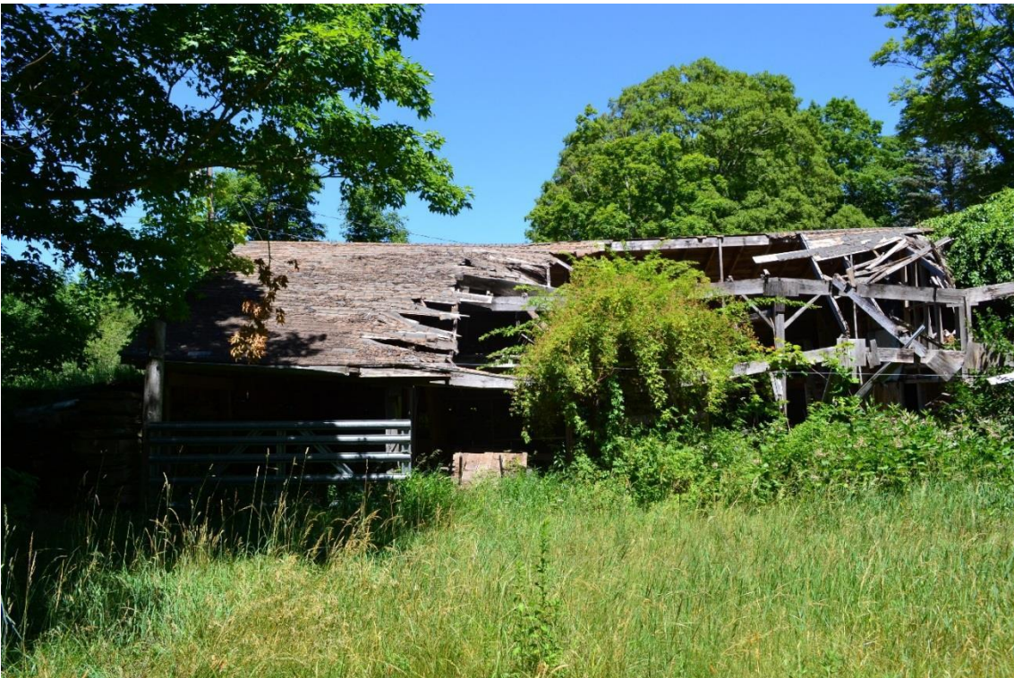
Photograph 10. Looking north at the western end of the barn (James Sexton, Tetra Tech, June 30, 2016).
