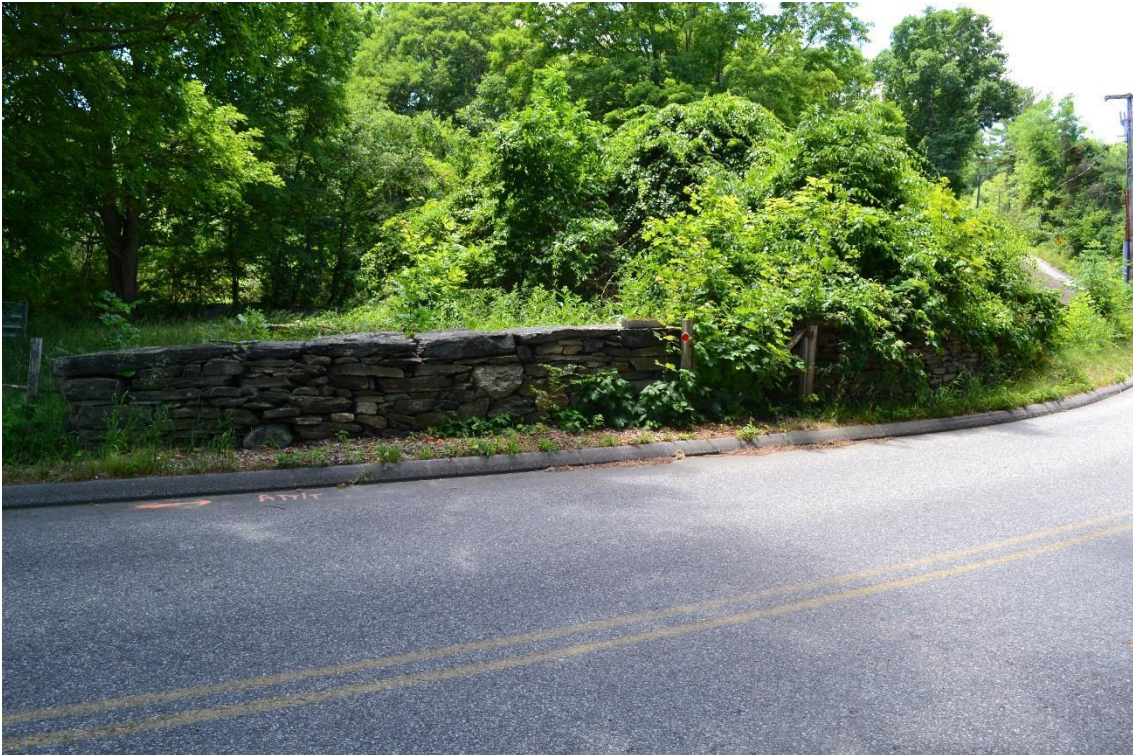
Photograph 13. Looking south at the stone wall to the east of the barn (James Sexton, Tetra Tech, June 30, 2016).
