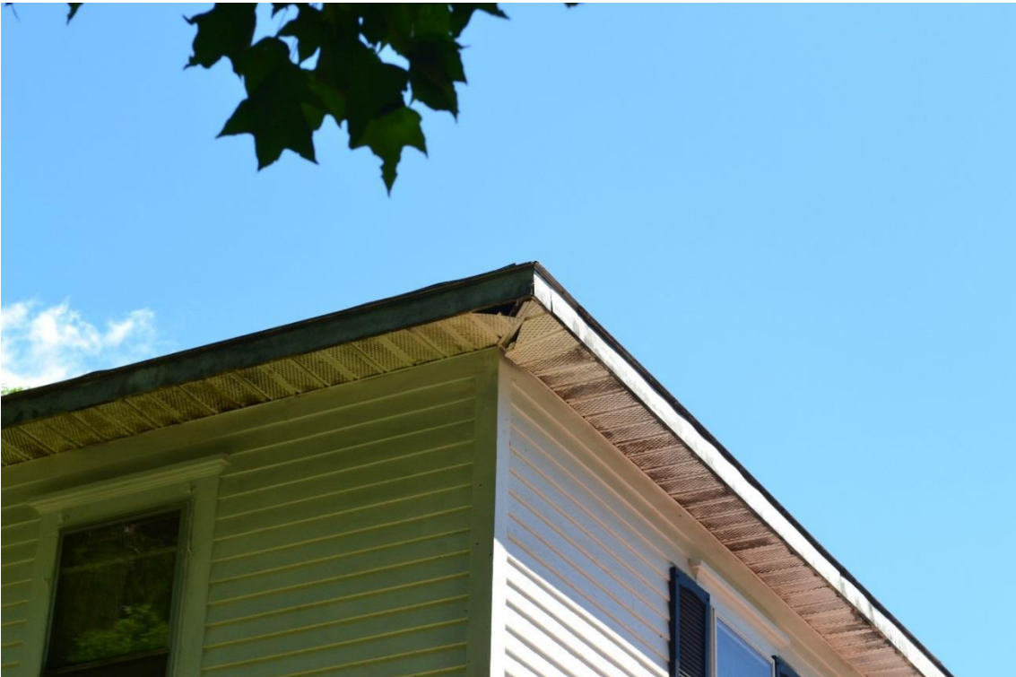
Photograph 6. Detail of the cornice at the southwest corner of Sorrow House (James Sexton, Tetra Tech, June 30, 2016).
