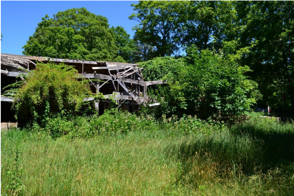
Photograph 11. Looking north at the western end of the barn (James Sexton, Tetra Tech, June 30, 2016).
