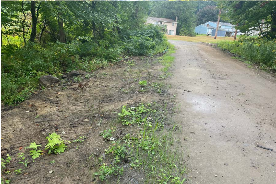
Photo 1: View of access entrance off Phillane Drive. Note surface stabilization needed when feasible.
