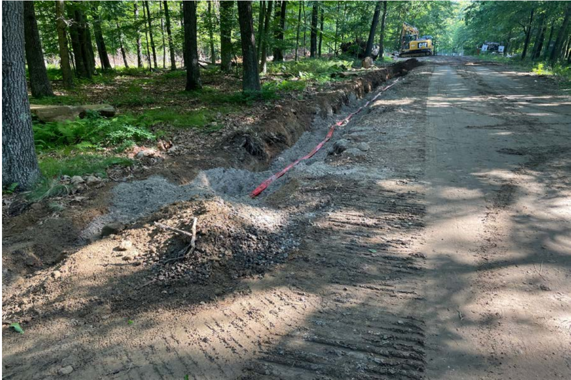
Photo 3: View of ongoing utility trench work along access road north of entrance.
