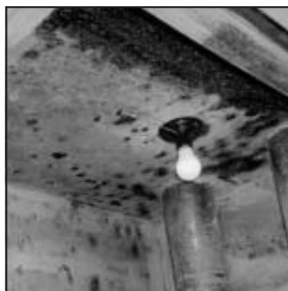
Photo 2. Ceiling of furnace room. Black is Stachybotrys .
