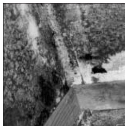
Photo 4. Close-up photo of Stachybotrys on the wall in Photo 3.
