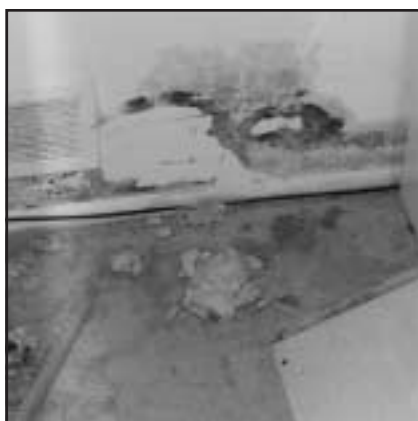
Photo 1. Large mushrooms on carpet. Furnace room is behind the return grille on the wall. Black on wall is Stachybotrys .
