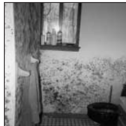
Above, Water wicked up bathroom wall causing growth.
