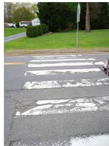
Faded crosswalk at school exit driveway.
