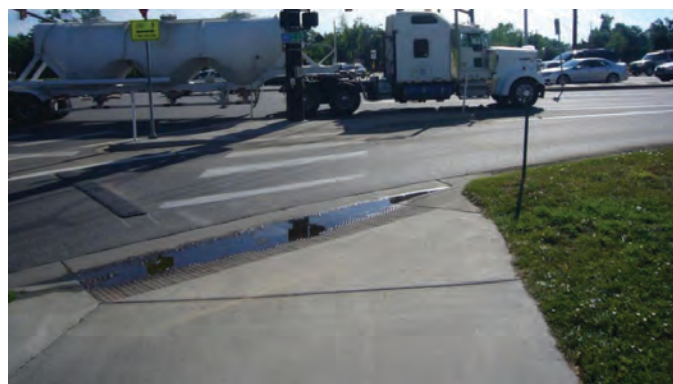
Figure 5-9. Example of a poorly aligned crosswalk at a CTL.
