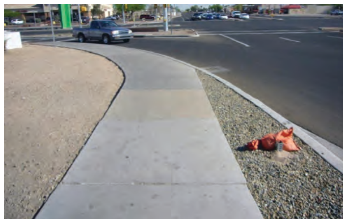
Figure 3-8. Sidewalk separation at a CTL not carried to the crosswalk.
