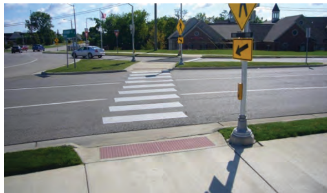
Figure 3-9. Roundabout crosswalk aligned too far to the left of the island landing.
