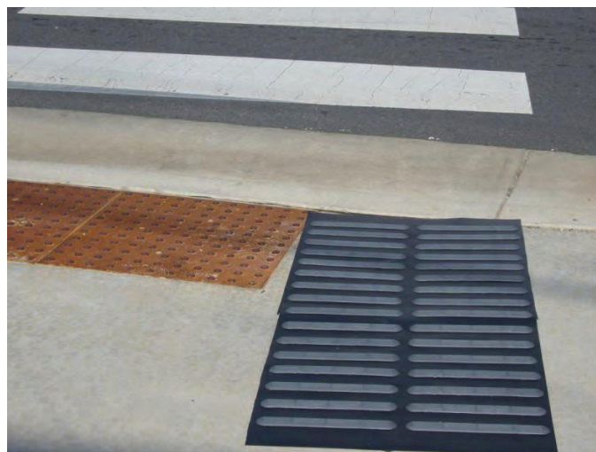
Figure 4-14. Experimental bar tile with bars perpendicular to the direction of the crosswalk.
