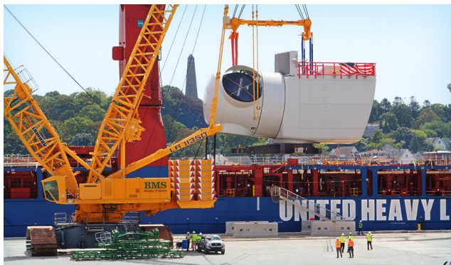
August 2023: Workers unload a 600-ton offshore wind nacelle at State Pier Terminal in New London. Photo credit: Quinn & Hary Marketing/Public Relations
