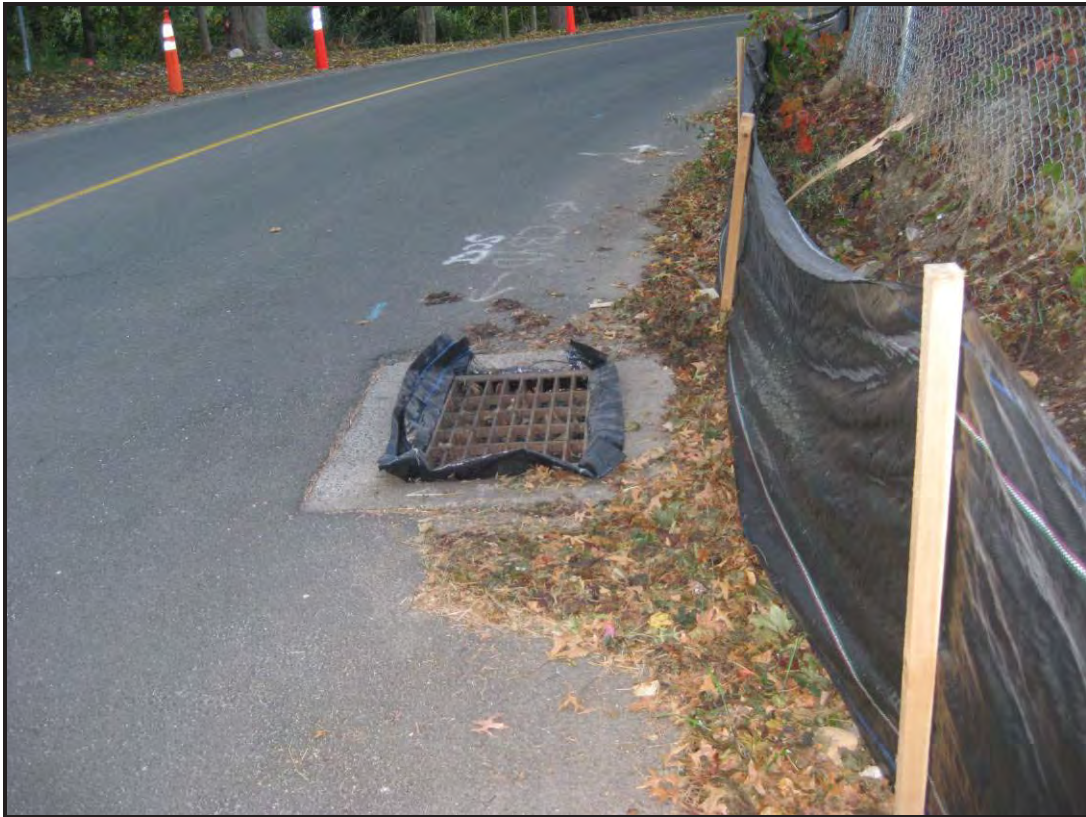
Catchbasin protected from sedimentation by filter fabric.
