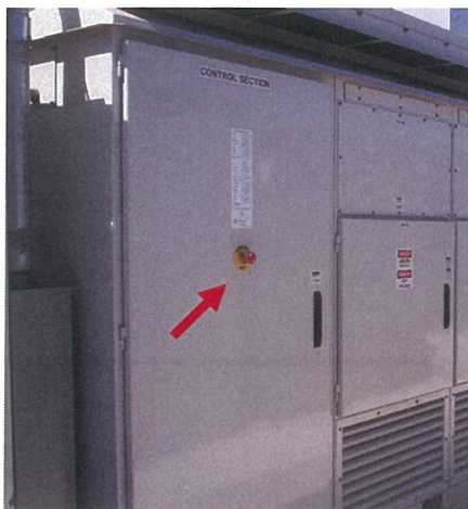
Electrical Balance of Plant Power Conditioning Unit
