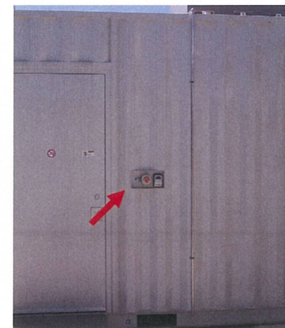
Skid 1, Electric & Controls / Water Treatment System Skid
