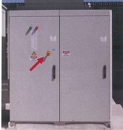
Tie Breaker Switchgear
