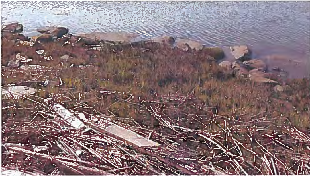
PHOTO 5: View of northwestern bank of watercourse 1 in vicinity of coastal jurisdiction line.
