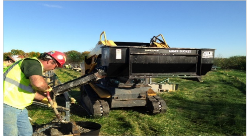
Bobcats with pouring buckets allow fast concrete installation on weight sensitive landfill caps: 20 men install 1.54MW per week
