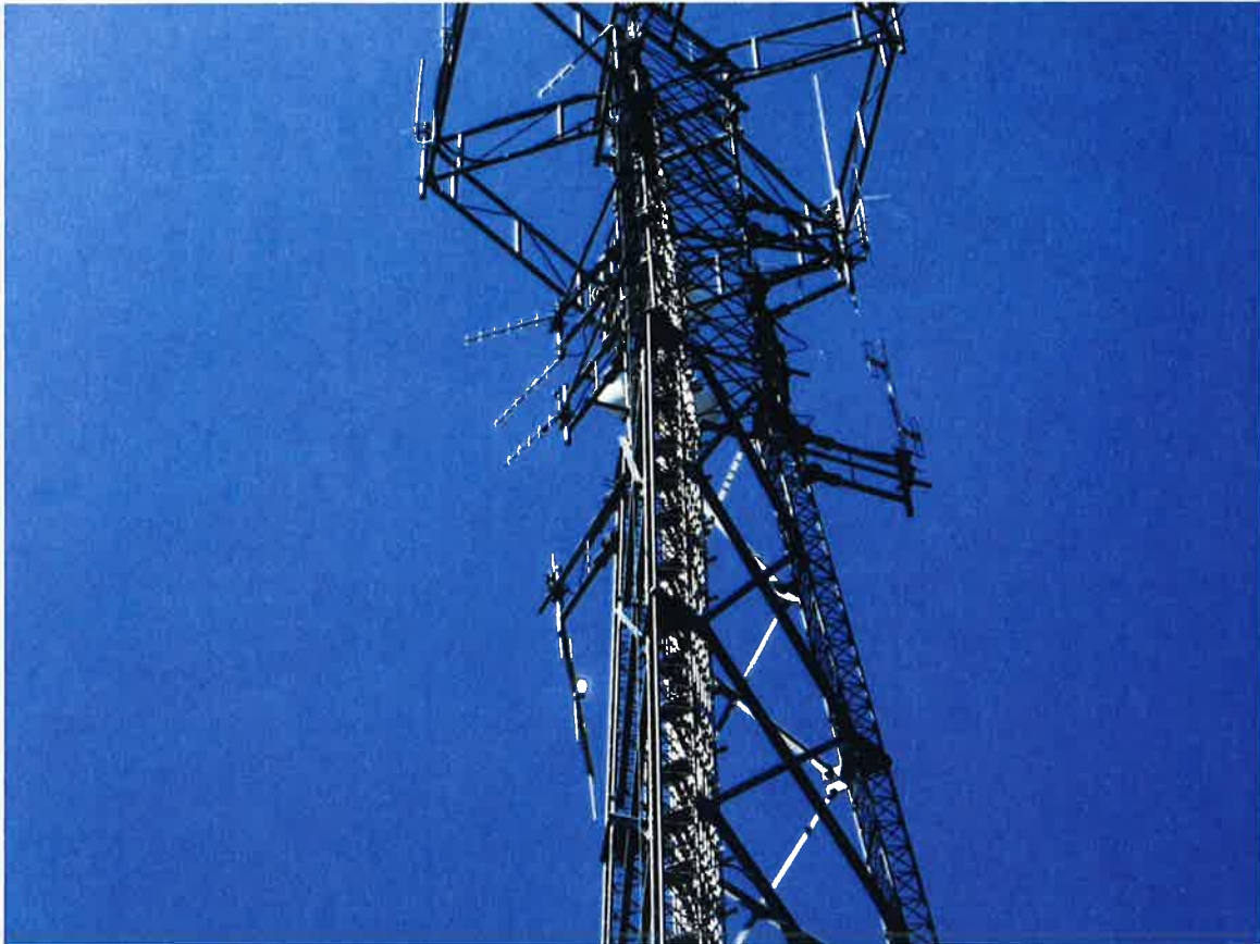
Photo 1: Photo illustrating the Tower with Appurtenances shown.
