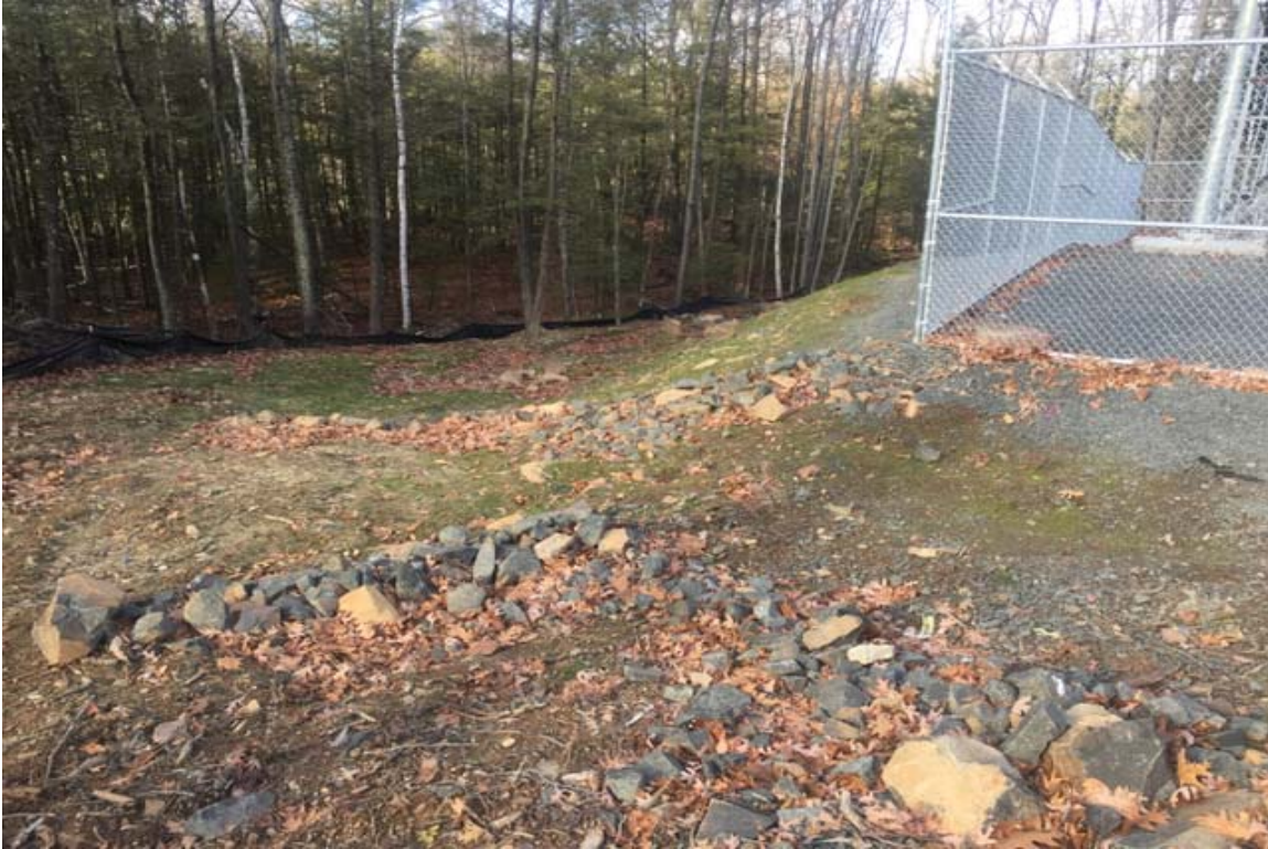
Photo 5: View of slope, drainage swale and south side of compound with germinated grass looking northwest.
