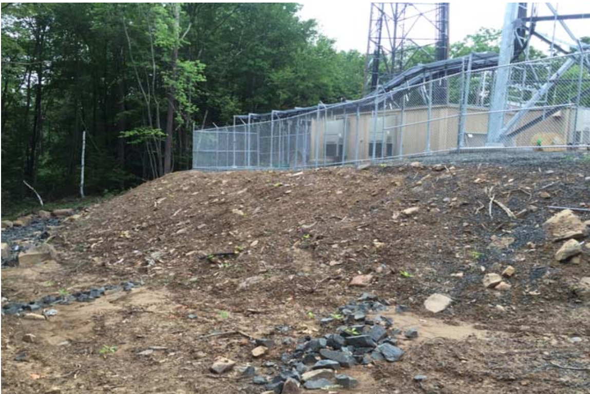
Photo 6: View of western slope looking north – requires installation of erosion blanket and seeding.
