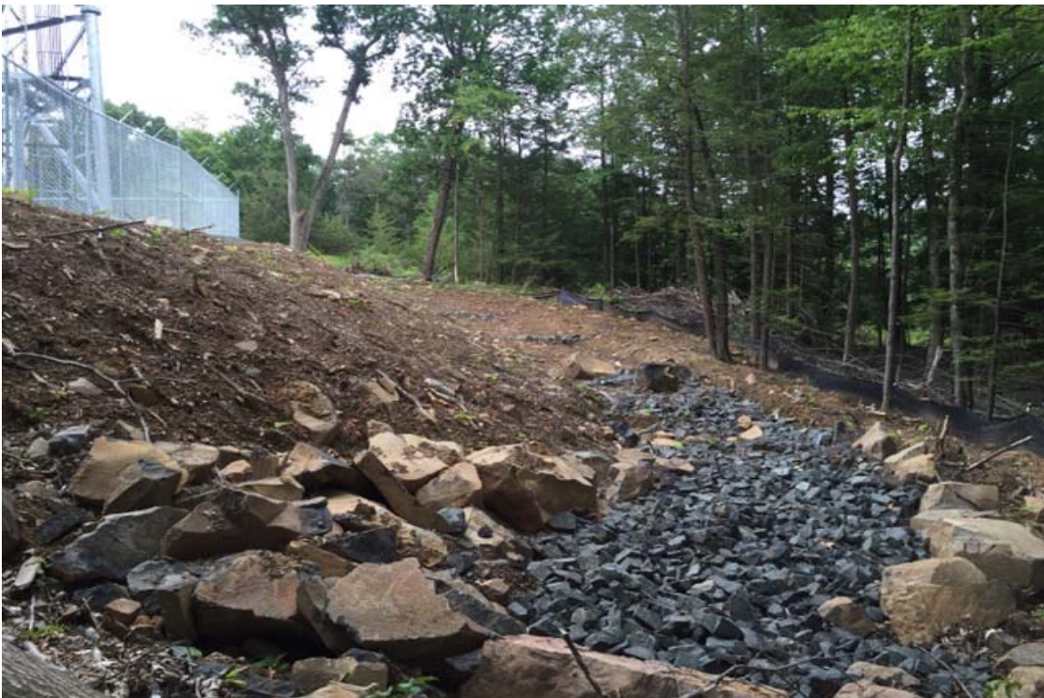
Photo 8: View of compound west slope and level spreader looking south – slope and drainage swale requires installation of erosion blanket and seeding.
