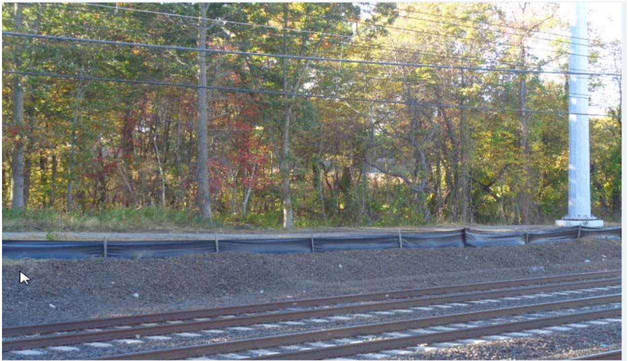
Access road with silt fence for Structure(s) 871S and 872S
