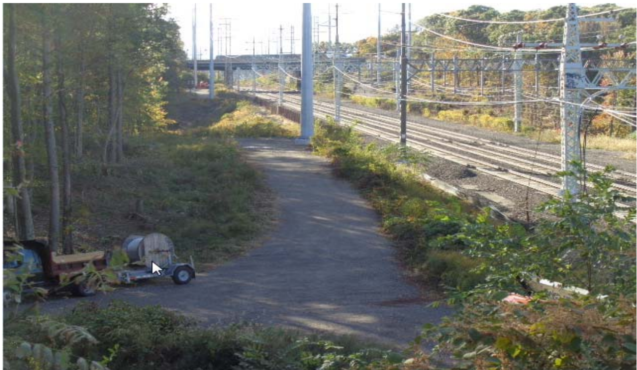
Access road along with erosion and sediment controls for Structure(s) 882S and 883S
