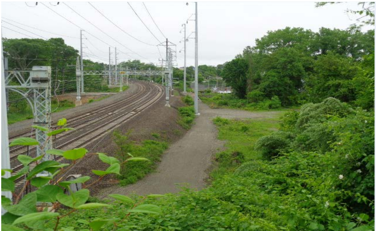
Structure(s) 884S, 885S and 886S Access Road, Work Pad(s) and E&S Controls
