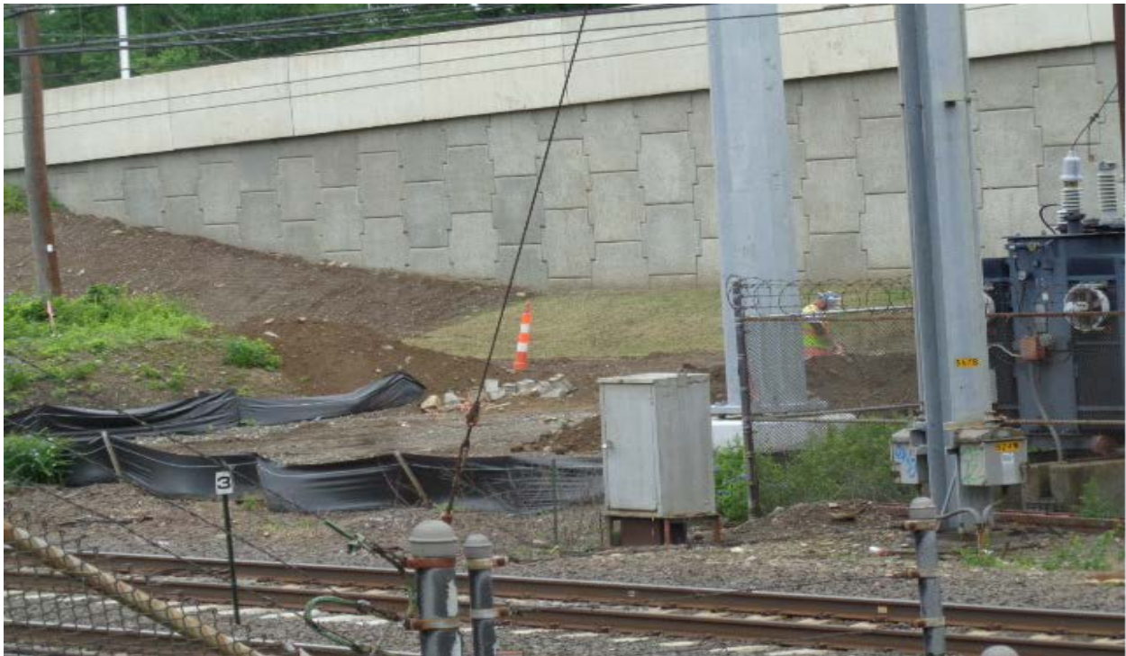
Structure 867S E&S Controls
