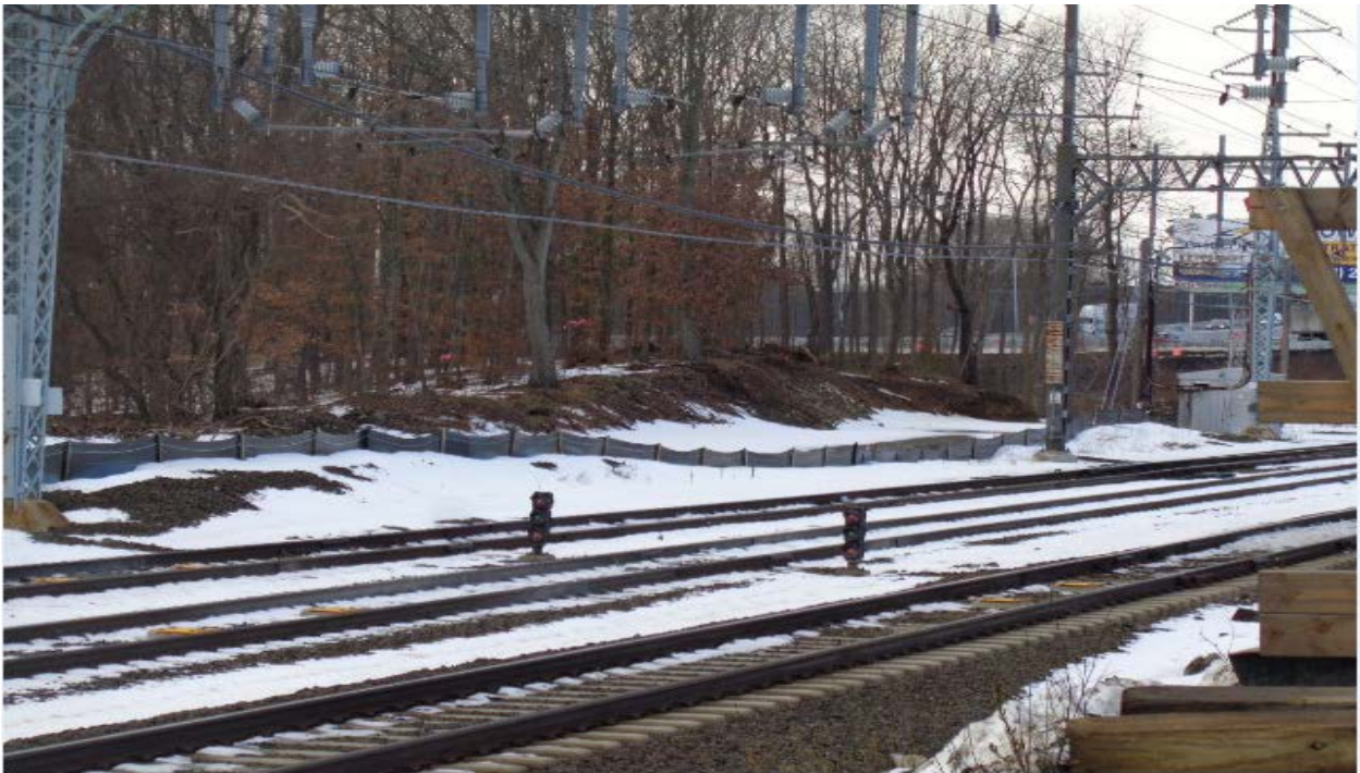
Access road, sediment and erosion controls between 871S and 872S
