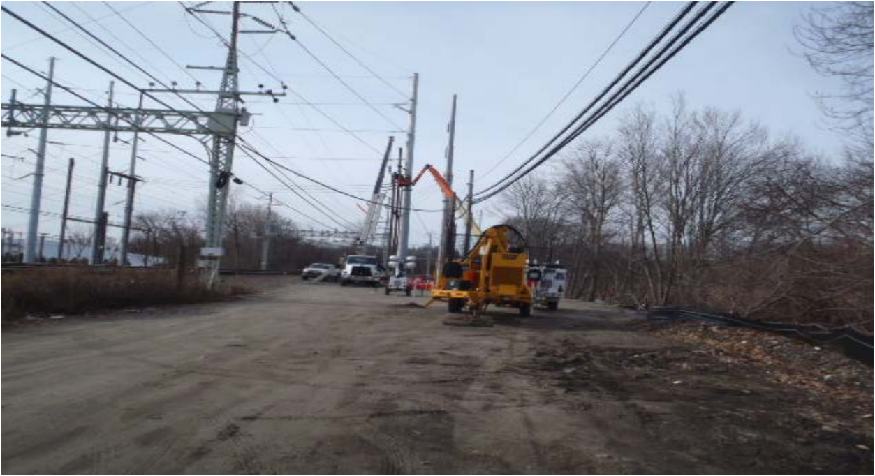
Structure 887N pull pad and sediment and erosion controls
