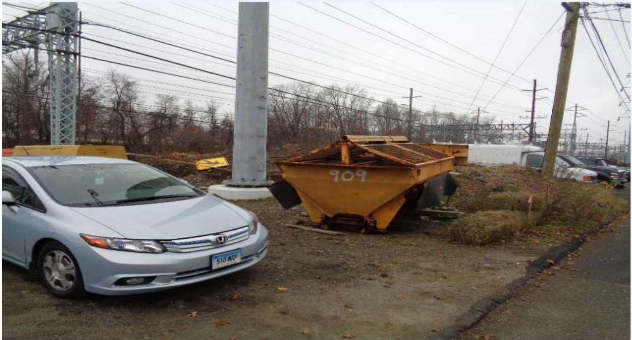
Structure 872N haybale barrier
