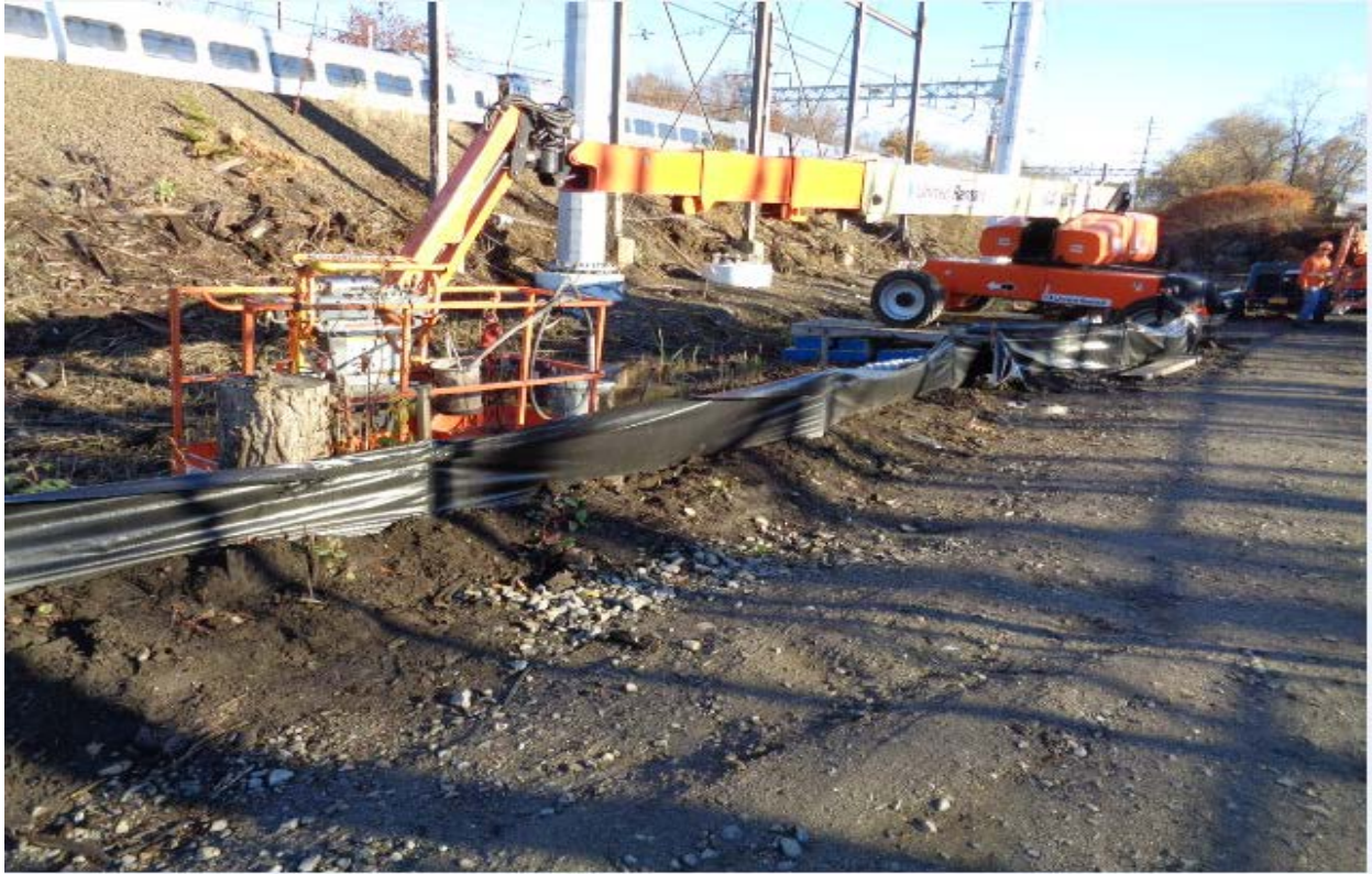
Structure 887S – temporary fill in wetlands along with erosion and sediment controls
