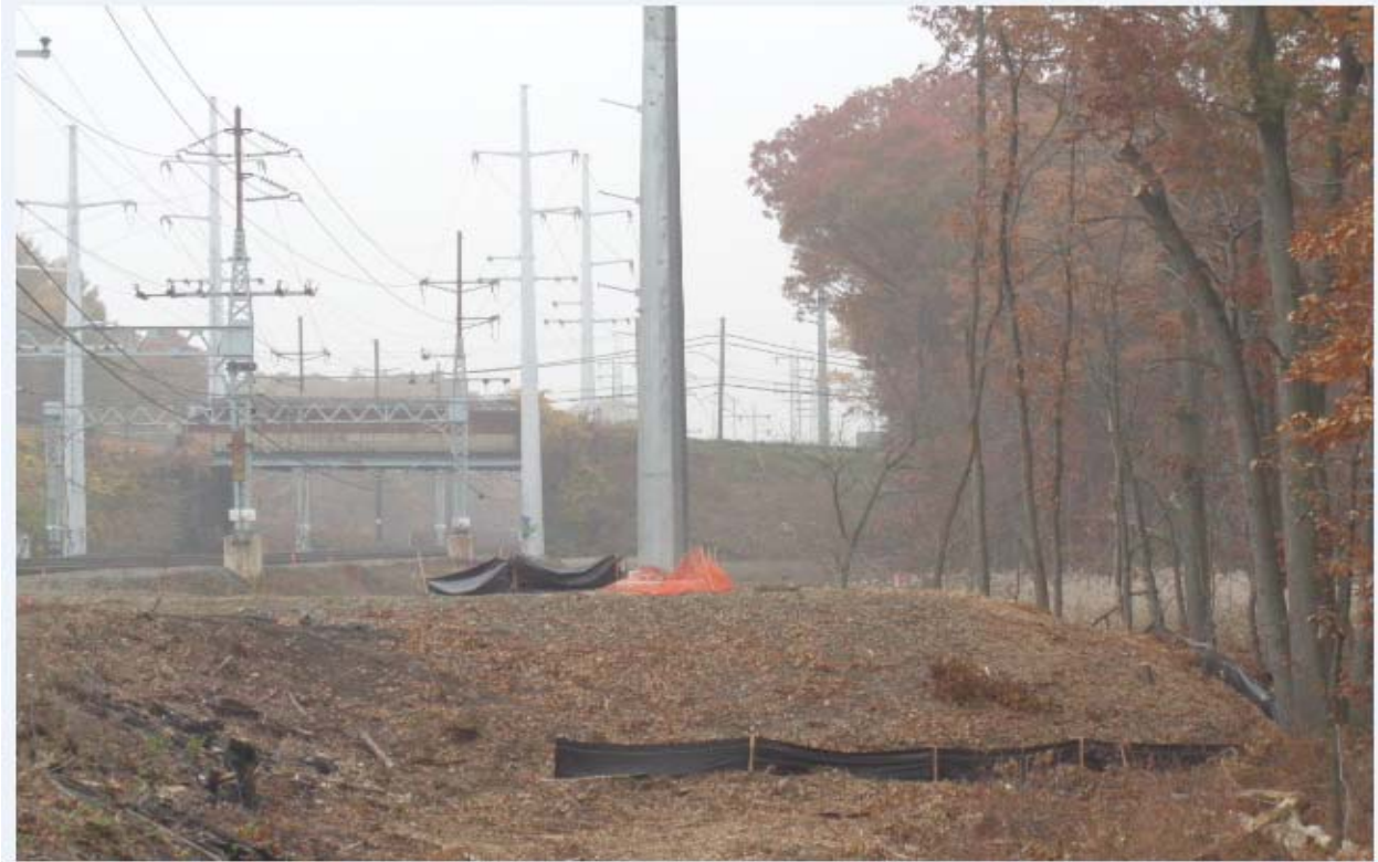
Structure 886N erosion and sediment controls
