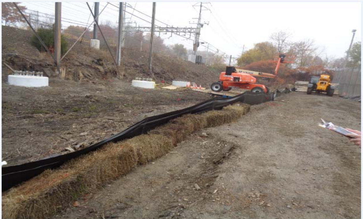
Structure 887S Erosion and sediment controls along with temporary fill (i.e., swamp mats)
