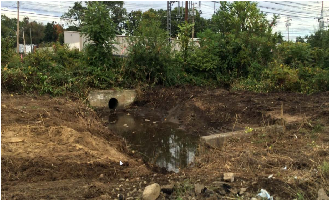
Trespassing Issue at culvert/wetland between 867S and 868S
