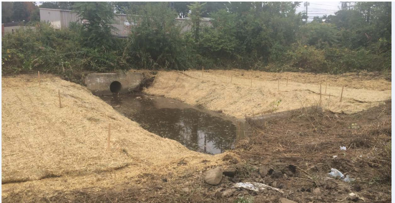
Restoration performed by UI and its contractors to culvert between 867S and 868S
