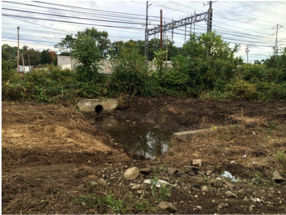
Wetland/culvert area vandalized, before stabilization
