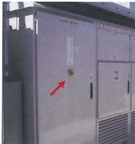
Electrical Balance of Plant Power Conditioning Unit
