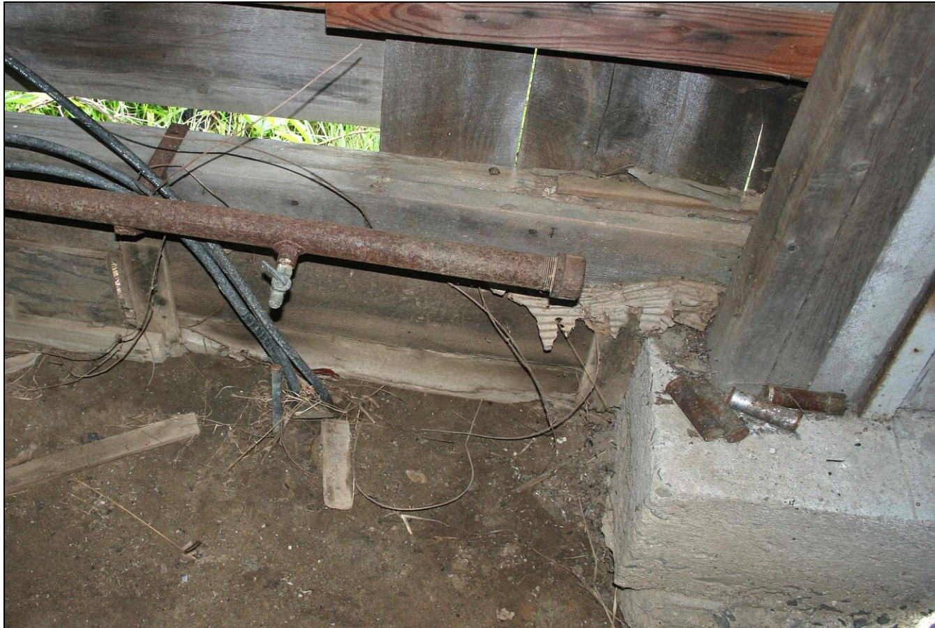
Photograph 74: Barn G (103), interior, detail of end of gas pipe, showing small valve.
