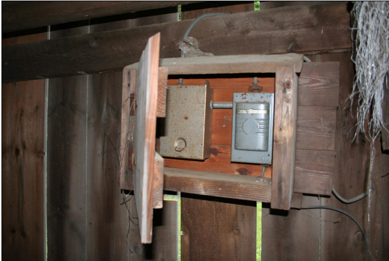
Photograph 38: Barn C (20), interior, detail of Trumbull Electric Company switch box.
