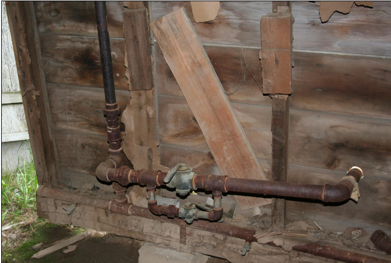
Photograph 66: Barn F (9), interior, detail of gas fittings.
