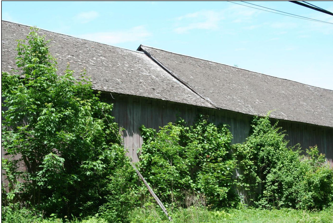
Photograph 8: Detail of break in roofline between 2-18 and 18 portions of Barn A, east elevation, camera facing west.
