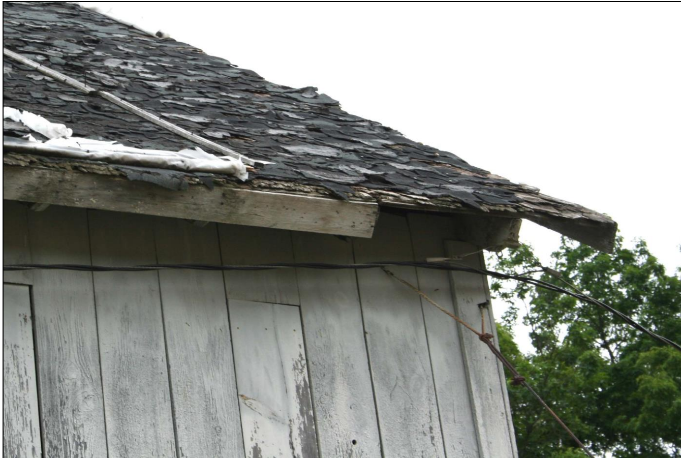
Photograph 34: Barn C (20), detail of roof edge, showing wood shingles beneath asphalt shingles.
