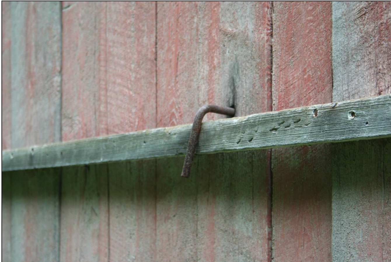
Photograph 10: Detail of rotating hook that secures operating bar in the closed position, Barn A (2-18/18).
