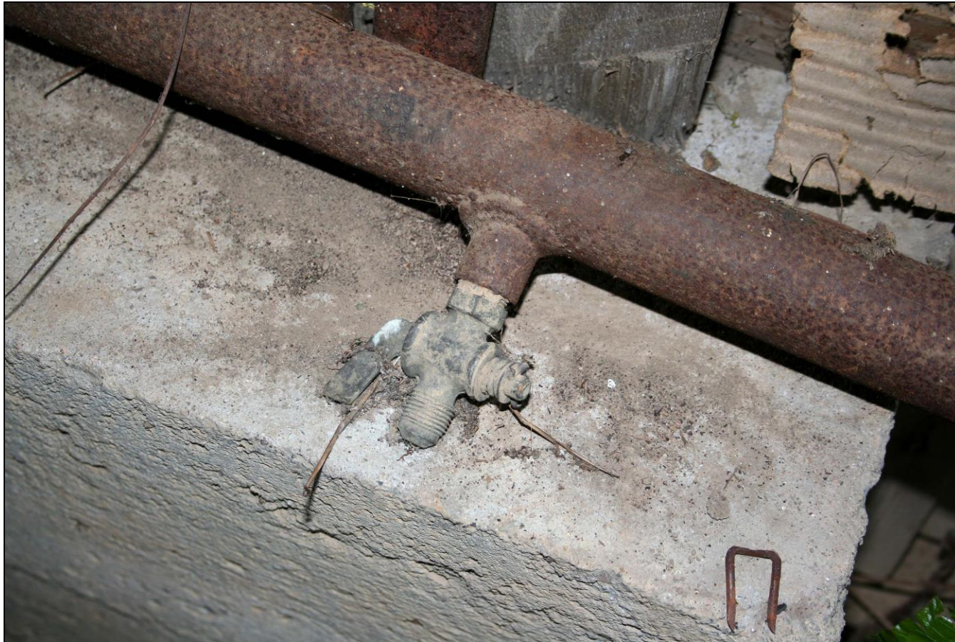
Photograph 83: Barn H (104), interior, detail of gas fitting.
