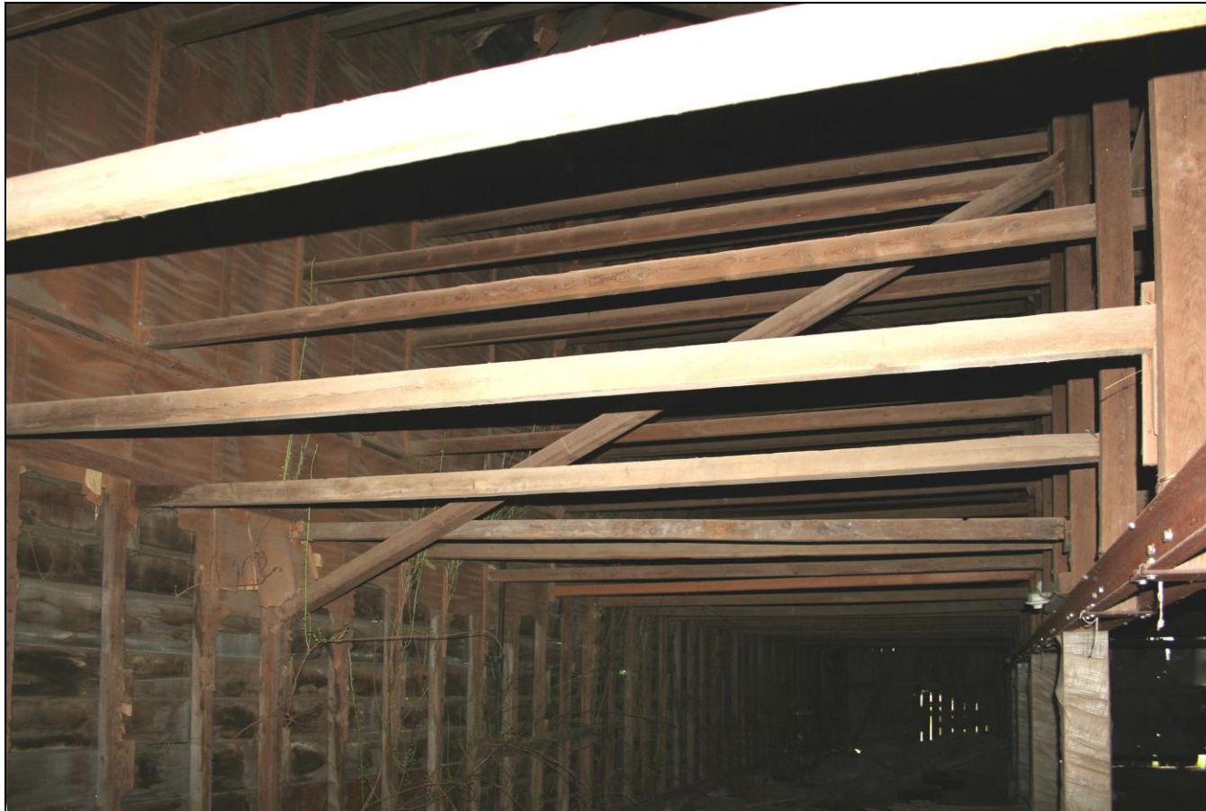
Photograph 94: Barn I, interior, detail of east side bay, showing diagonal wind brace.
