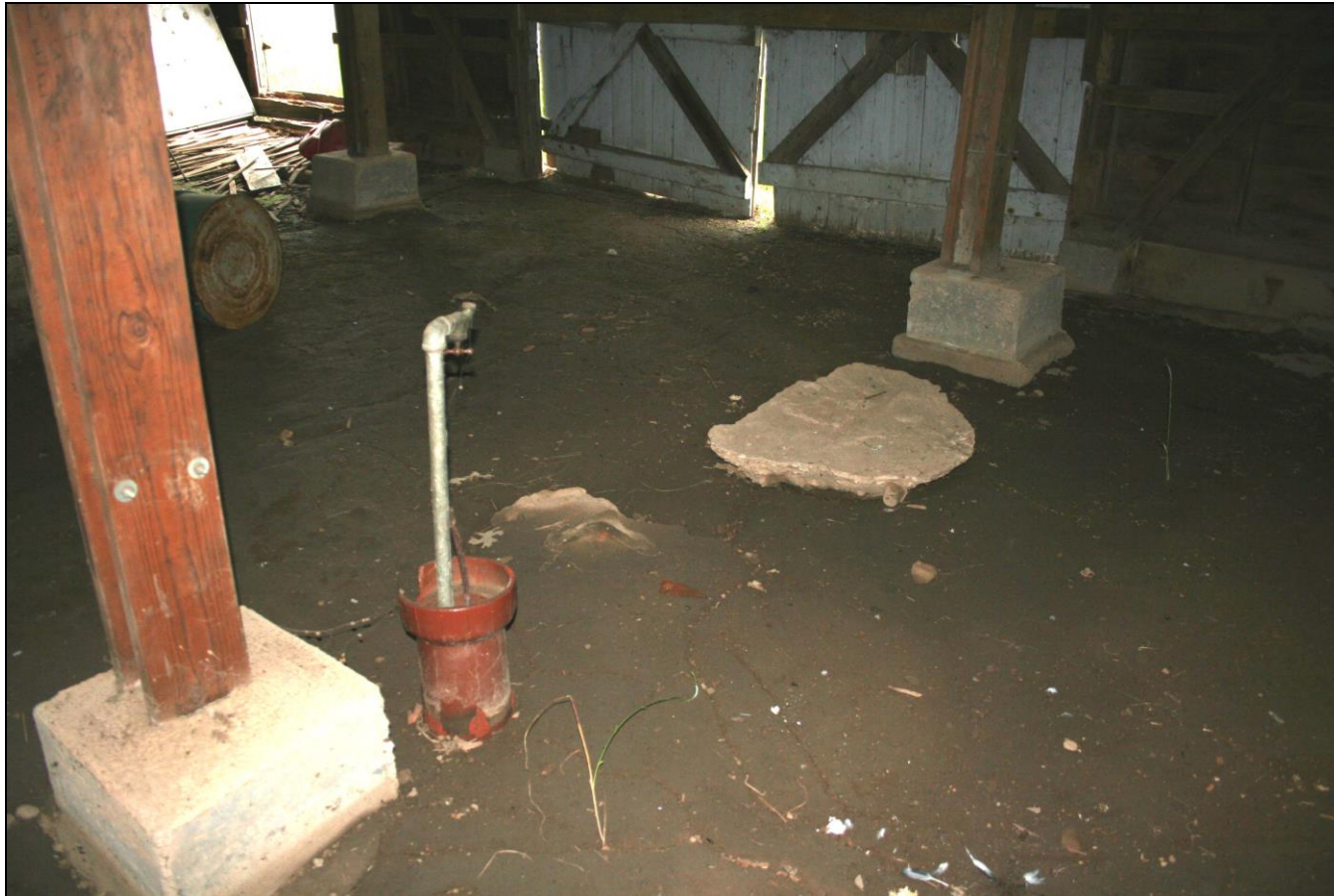
Photograph 134: Barn N (2-16), interior, detail of water spigot and remnants of footing for two intermediate posts.
