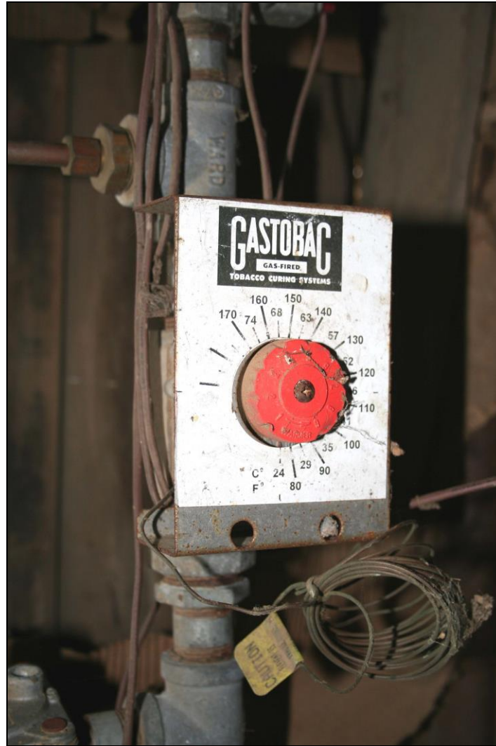
Photograph 50: Barn D (7), interior, detail of “Gastobac” gas thermostat.
