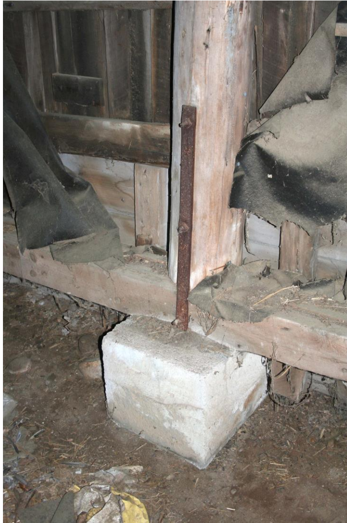
Photograph 15: Detail of method of anchoring post and sill to footing with iron strap, Barn A (2-18/18).
