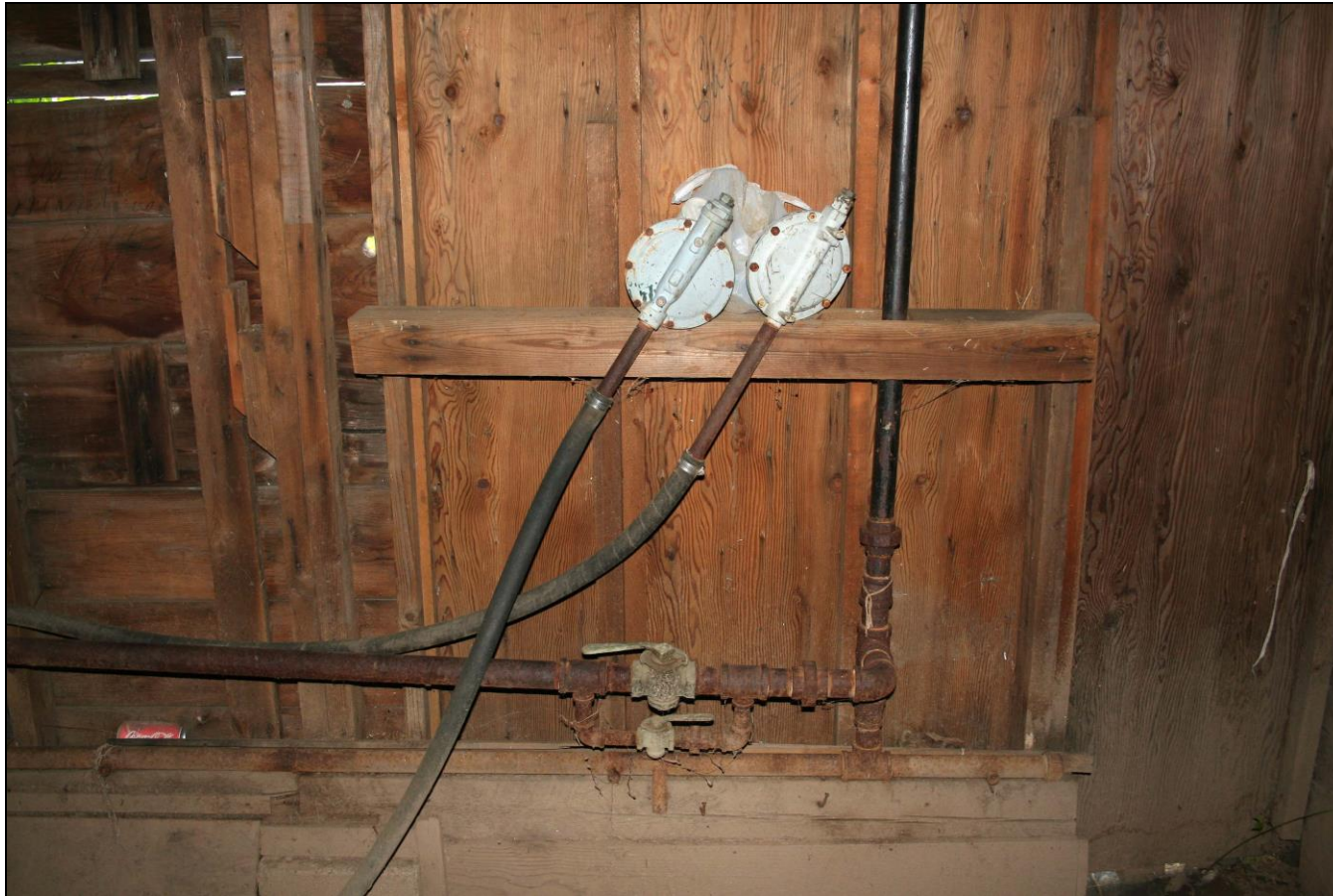
Photograph 136: Barn N (2-16), interior, detail of gas fittings and two gas regulators attached to rubber hoses.
