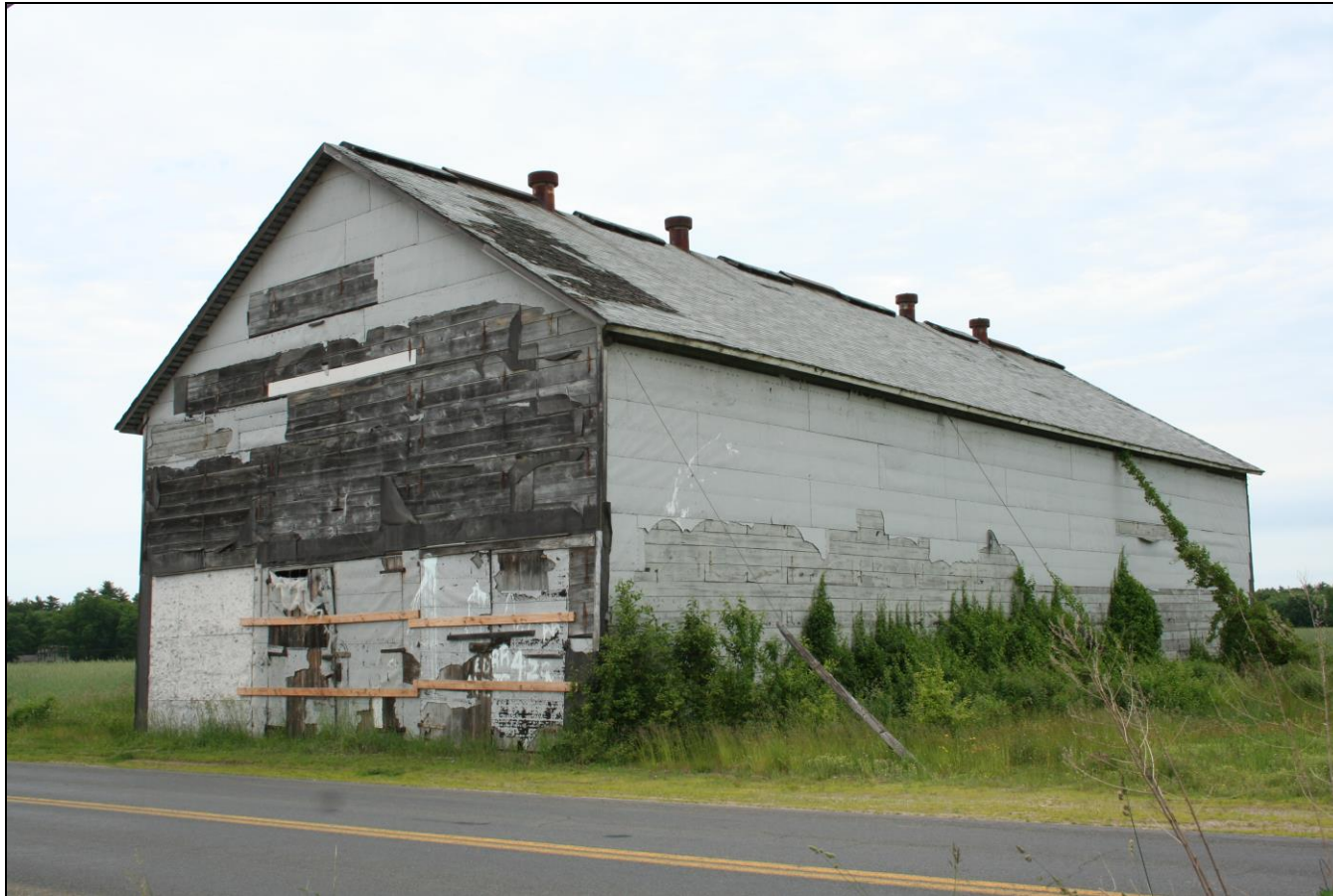
Photograph 88: Barn I (unnumbered) on north side of Firetown Road, south and east elevations, camera facing northwest.
