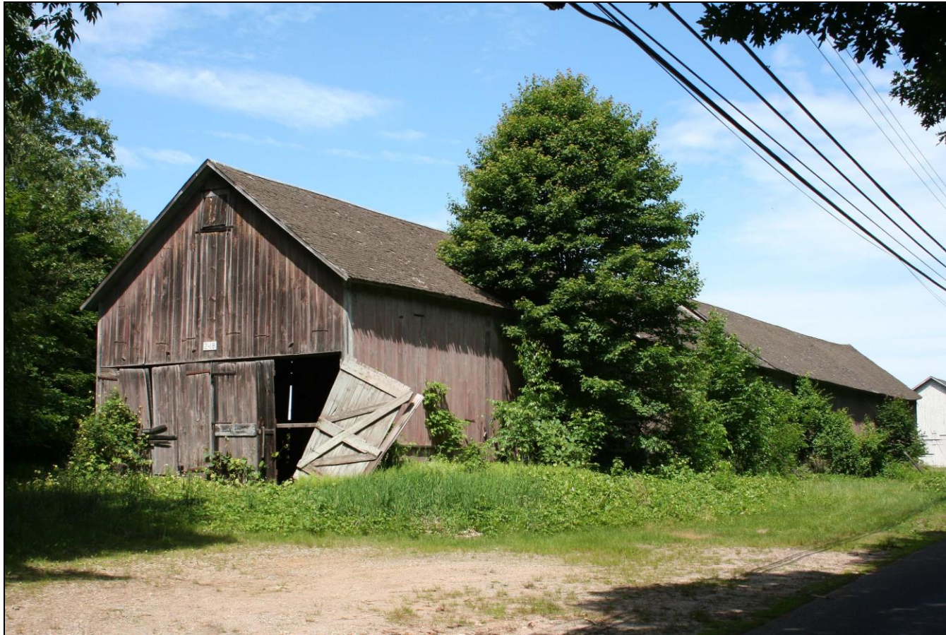
Photograph 5: Barn A, numbered 2-18 on its south end and 18 on its north end, south and east elevations, camera facing northwest.
