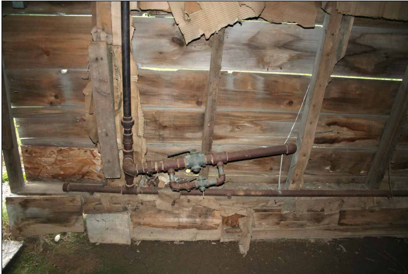
Photograph 56: Barn E (8), interior, detail of gas pipe and fittings.
