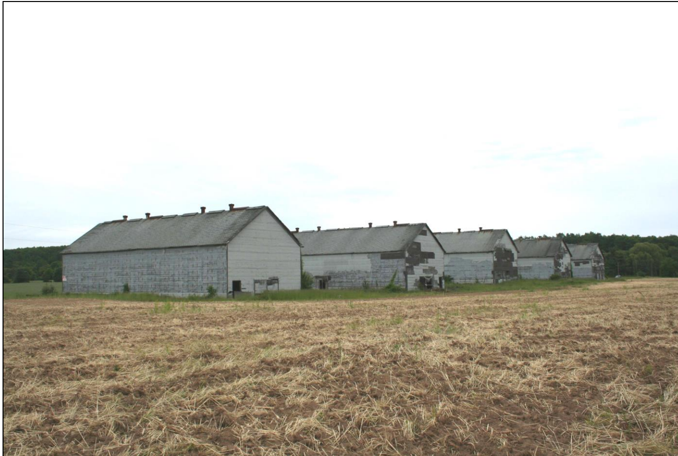
Photograph 86: Field side (south elevations) of barns on south side of Firetown Road, camera facing east; left to right, Barn N (2-16), Barn M (2-15), Barn L (2-14), Barn K (2-13), and Barn J.
