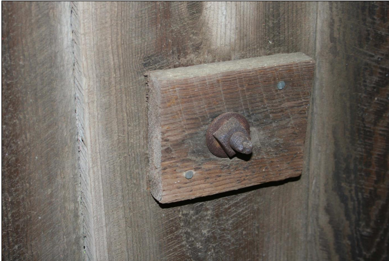
Photograph 11: Detail of the inside of the hook that secures the operating bar in the closed position, Barn A (2-18/18).
