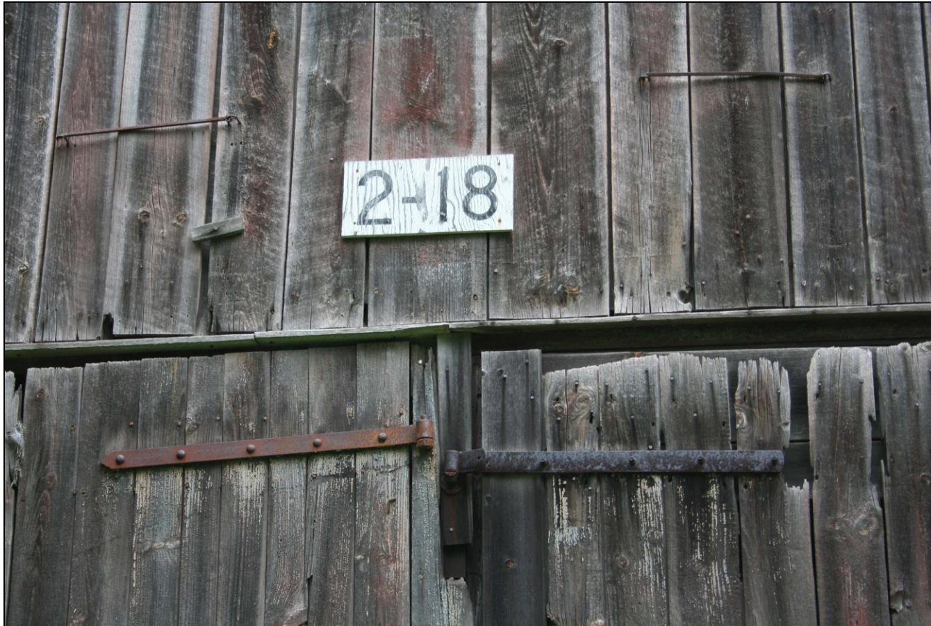
Photograph 12: Detail of number placard and strap hinges, south end of Barn A (2-18/18).
