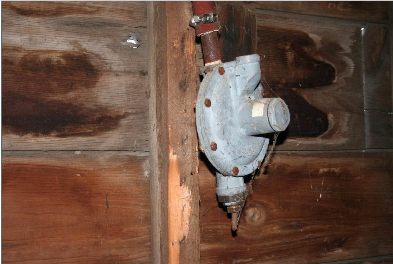
Photograph 125: Barn M (2-15), interior, detail of gas regulator attached to rubber hose.
