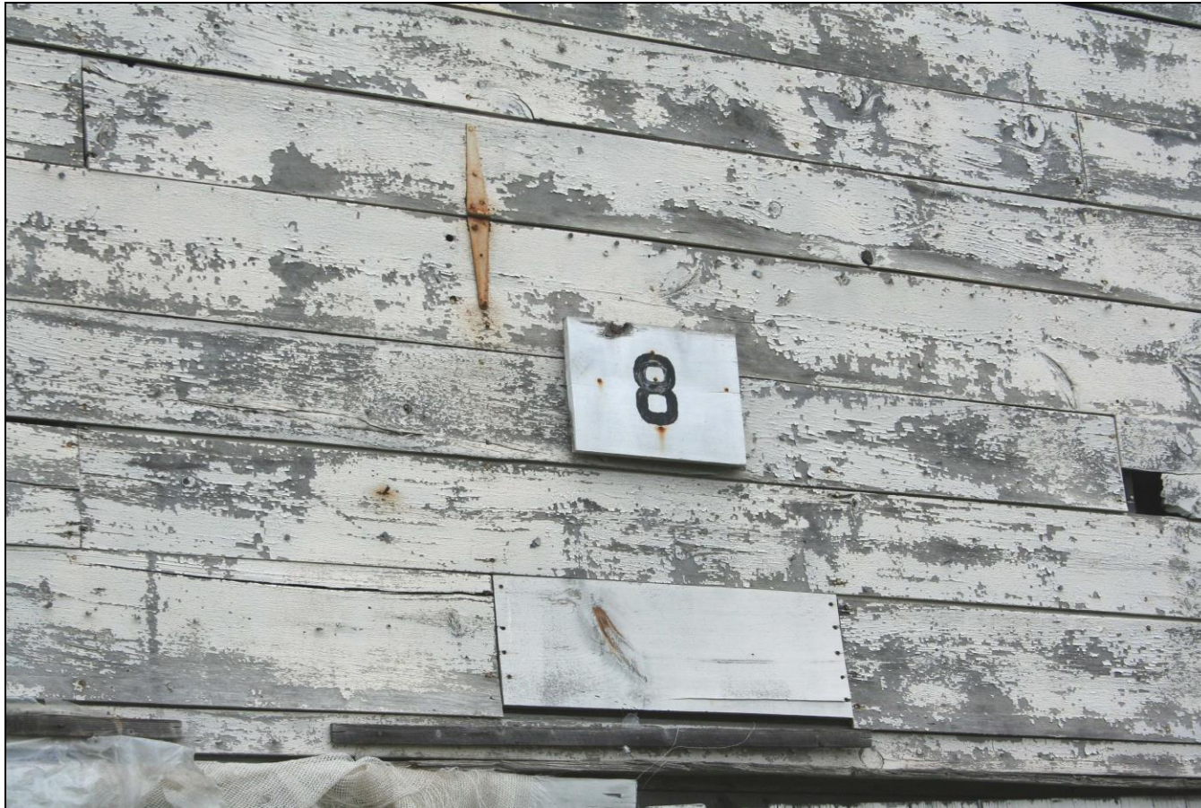
Photograph 54: Barn E (8), detail of number placard and hinged boards, south end, camera facing northeast.
