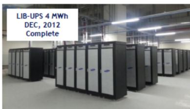
Shinhan Bank IDC Center in Jukjeon, Korea
