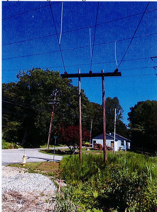
Existing wood H-frame structure 7020 1/2 with underbuilt "flying" tap design
