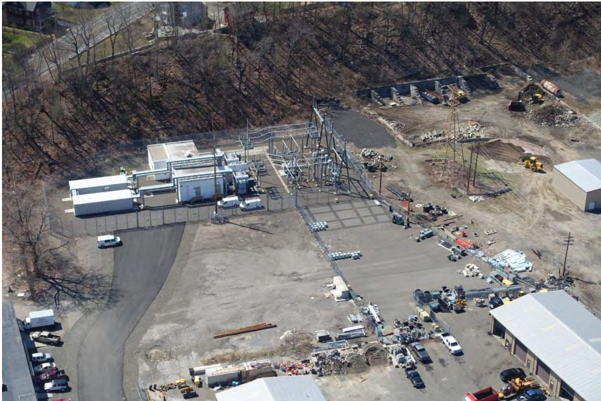
Figure A-1: Existing Ansonia Substation
