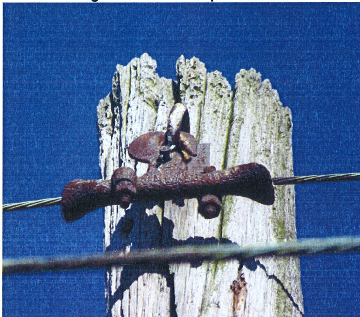
Figure H- 2 Pole-Top and Hardware Condition
