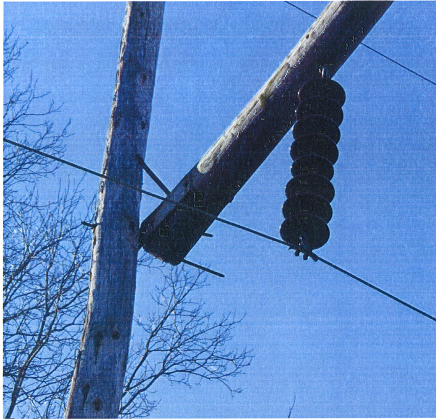
Figure H- 3 Pole and Cross Arm Condition
