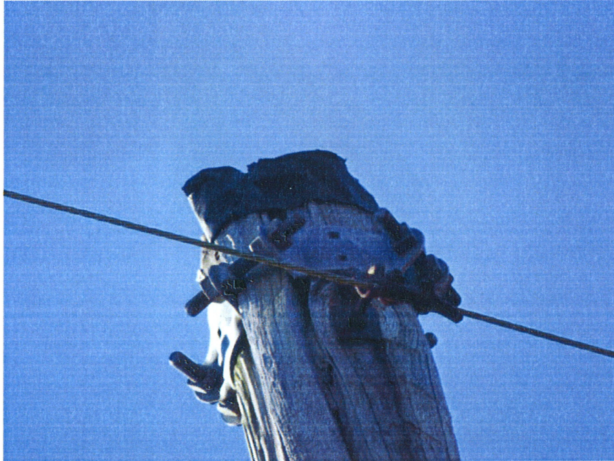
Figure H- 1 Pole-Top Condition
