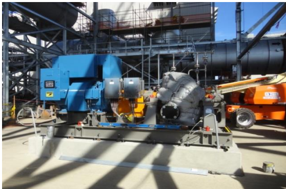
Set Condensate Pumps
