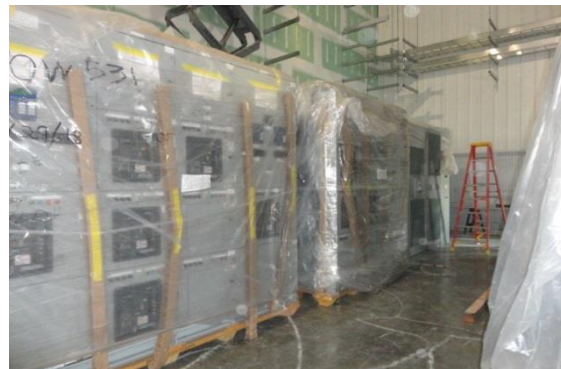
Switchgear in General Service Building
