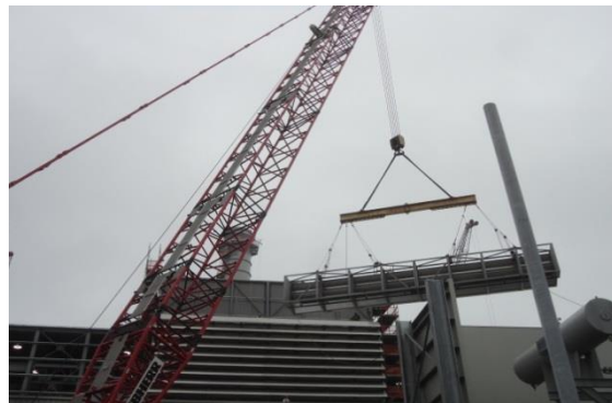
CT Air Inlet Hood Section
