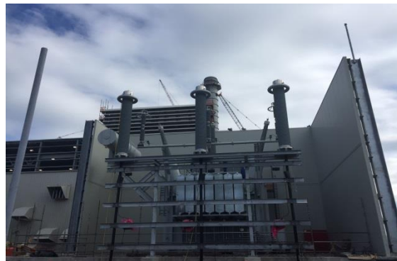
CTG 345kV HV Potheads
