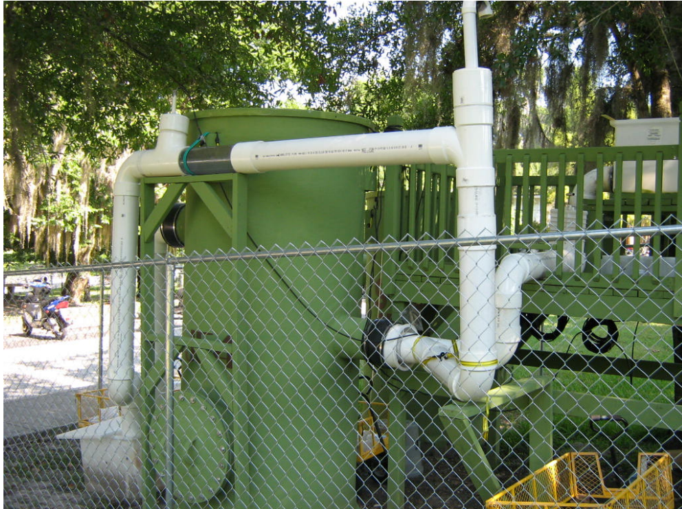
Figure 6 Photo of field test set-up for the Jellyfish ® Filter JF4-2-1. Below-deck inlet pipe enters the right side of the vessel and outlet pipe (invert at deck level) exits the left side of the vessel. External bypass piping has invert of horizontal section 18 inches above deck level.
