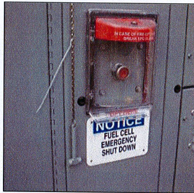
Figure 1: Emergency Power Off Button
