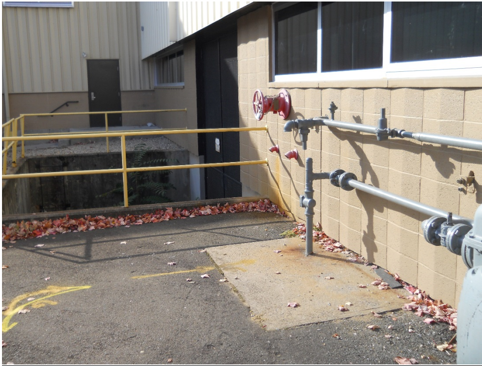
EXISTING GAS METER AND ELECTRICAL TRANSFORMER VAULT: SOUTH TO PROPOSED FACILITY
