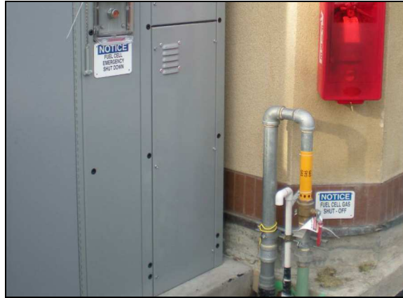
Figure 3: Manual Natural Gas Valve
