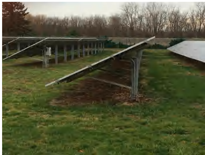
Figure 22. Existing solar panel array in Galstonbury, CT.
