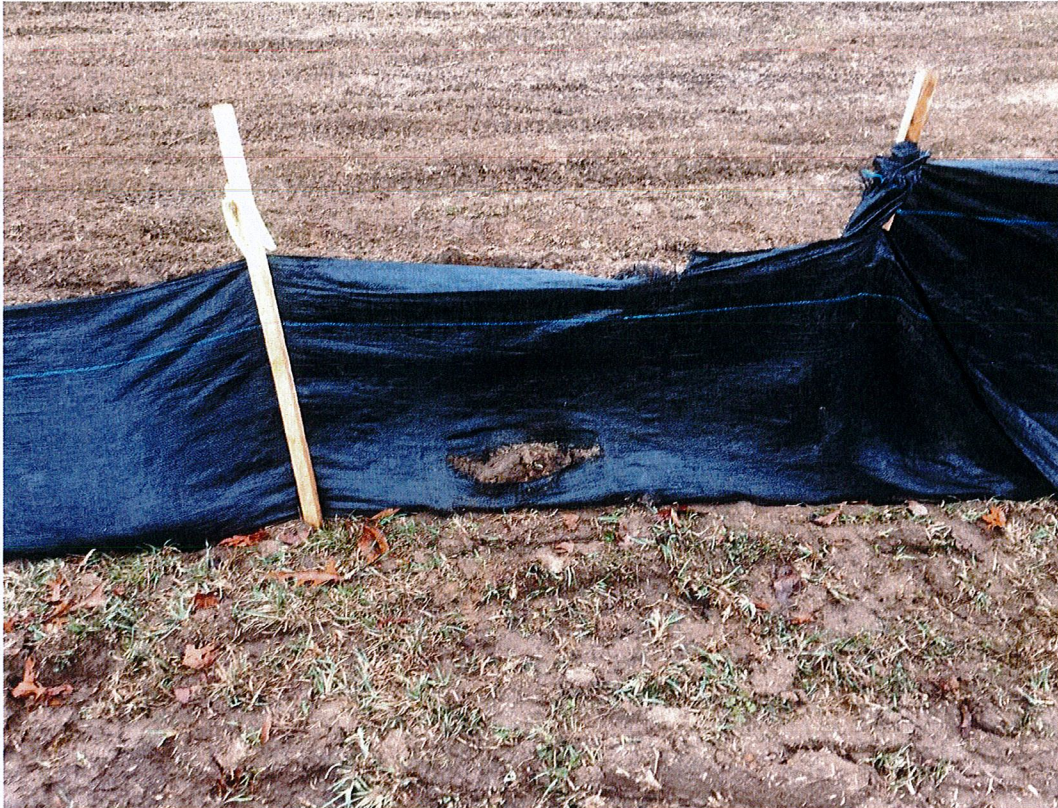
Photo 5: View of CA#4, gap in silt fencing.
