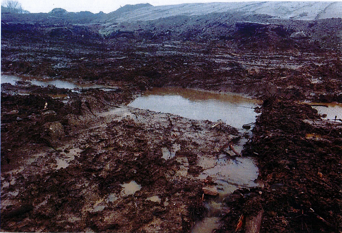
Photo 3: View of breach in diversion channel to sediment basin SB-3 looking north.
