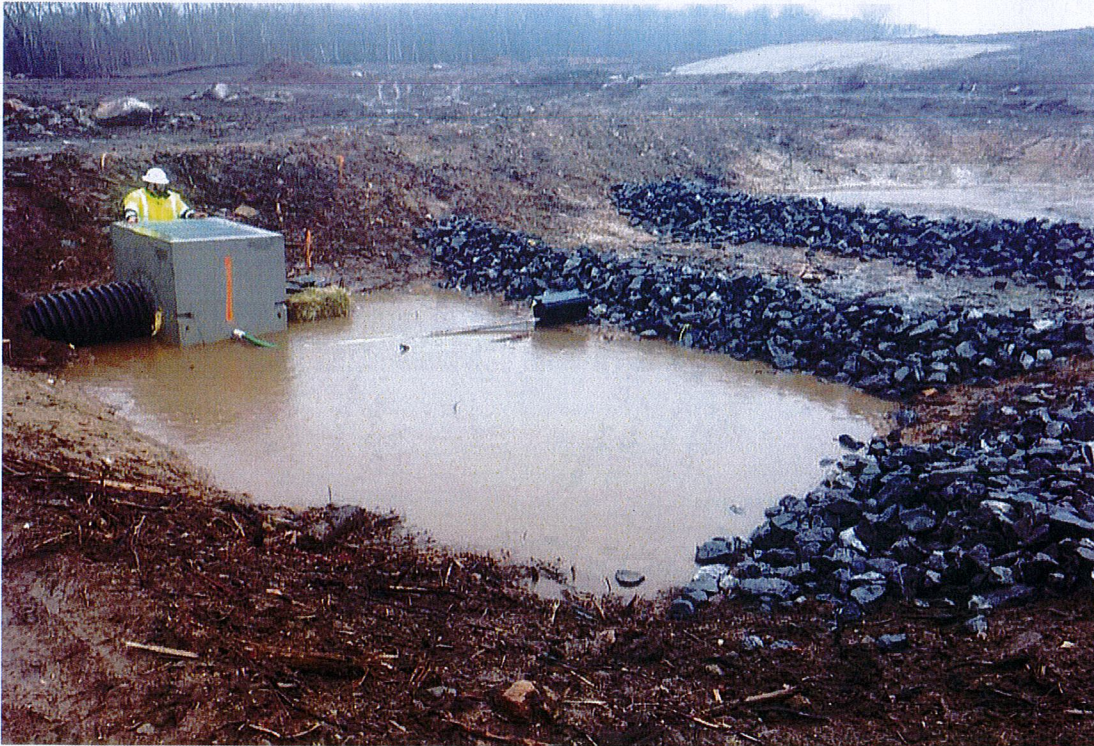
Photo 5: View of temporary sediment basin SB-3.
