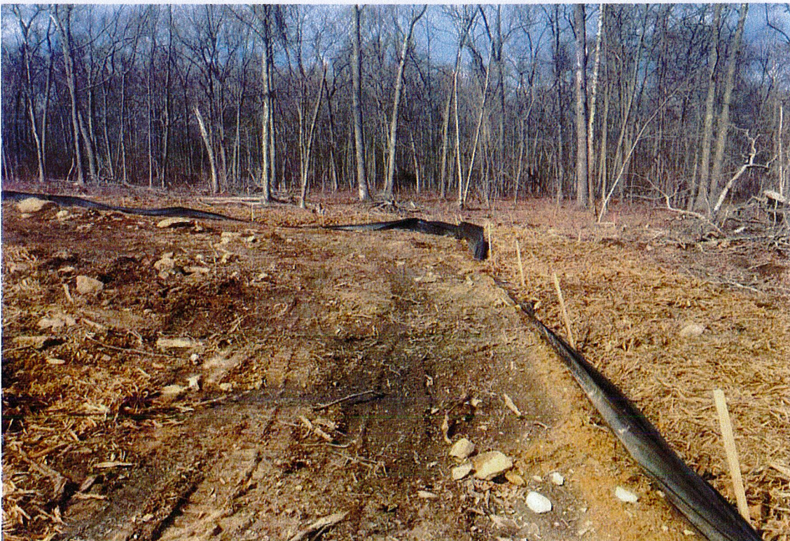
Photo 6: View of CA #7, silt fenced knocked over.
