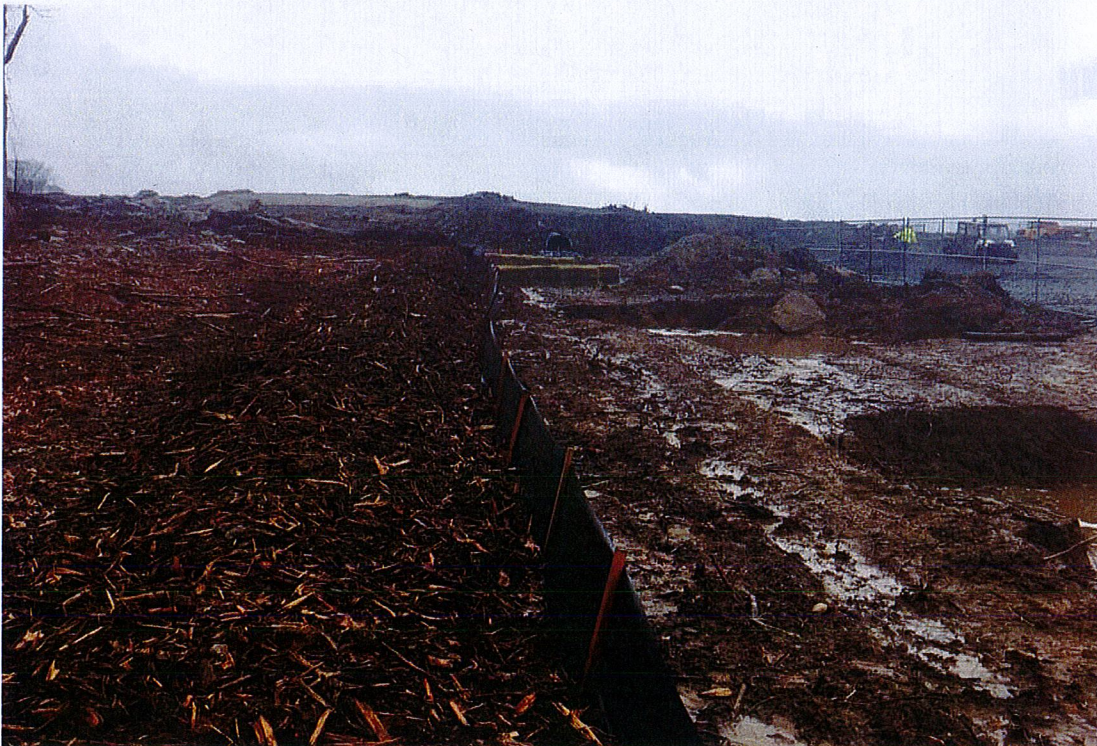
Photo 6: View of perimeter controls and primary flow path out-letting from temporary sediment basin SB-3 looking north.
