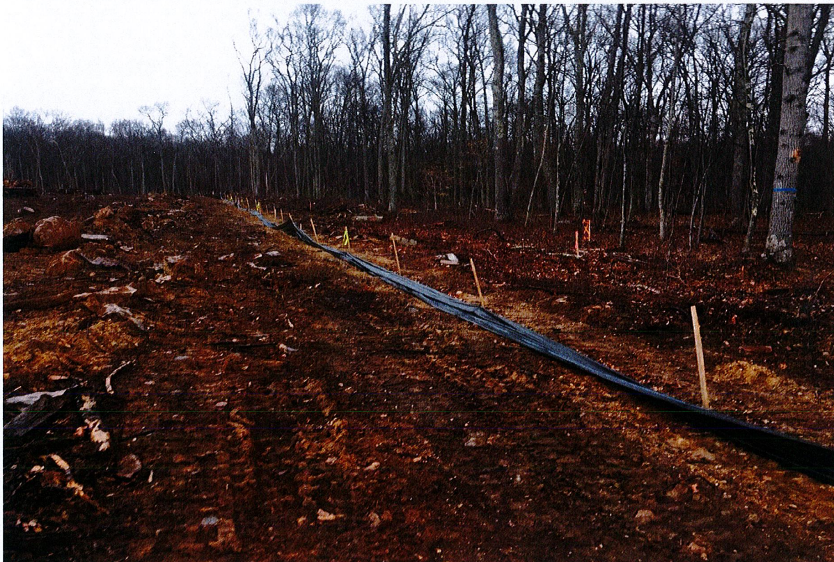
Photo 6: View of previously identified silt fence repair (CA#4) in northeast corner of project.
