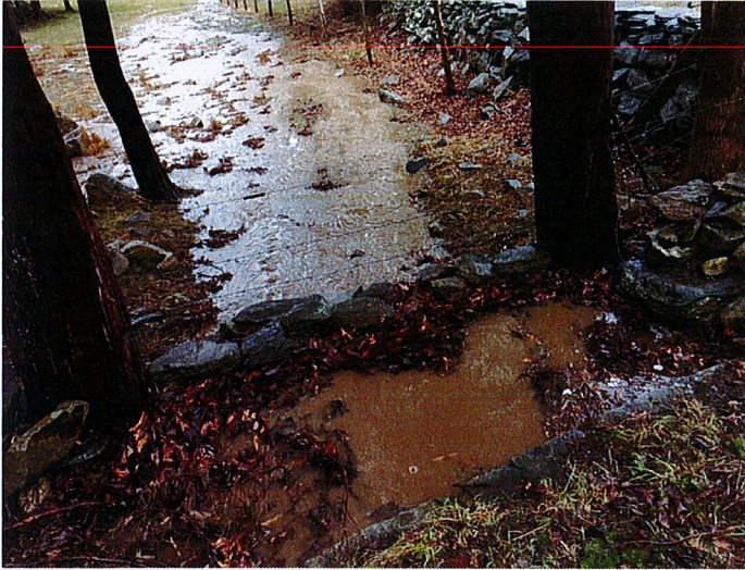
Culvert discharge onto Mr. Rainville's property.
