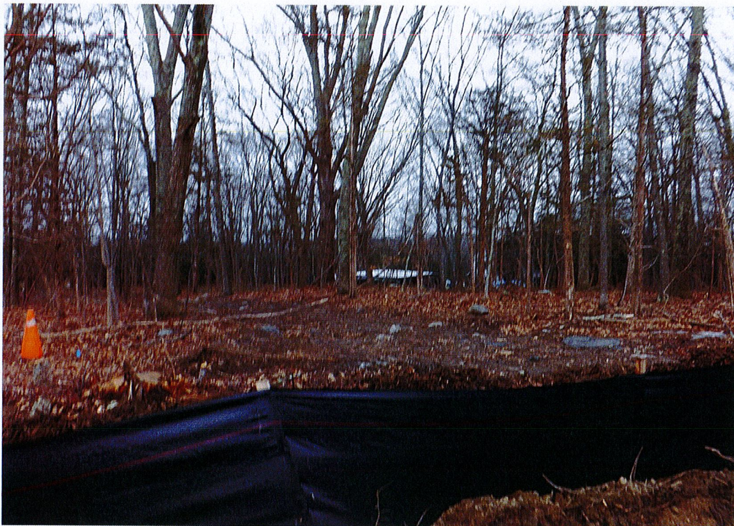
View of Silt Fence (on subject property) and Cone Depicting Mr. Bates' Property – View facing west
