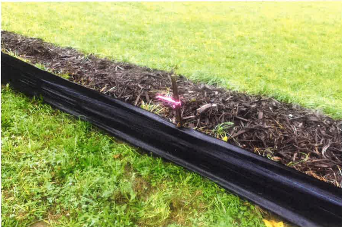
Photo 6: View of silt fence break needing repair.
