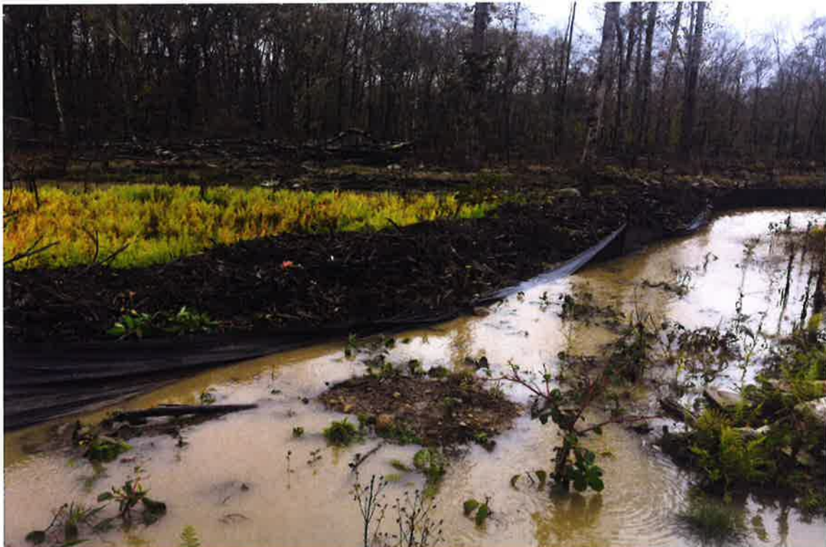
Photo 4: View of the silt fence needing repair looking east.
