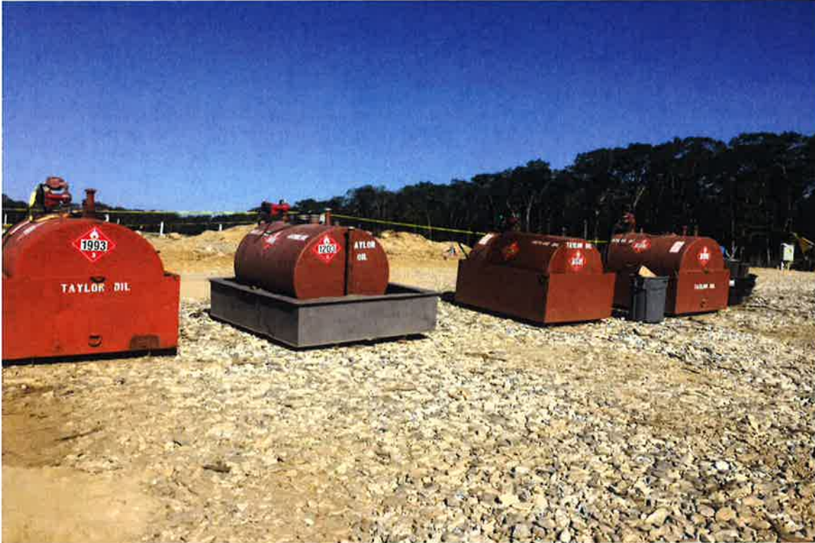
Photo 5: View of fuel storage.
