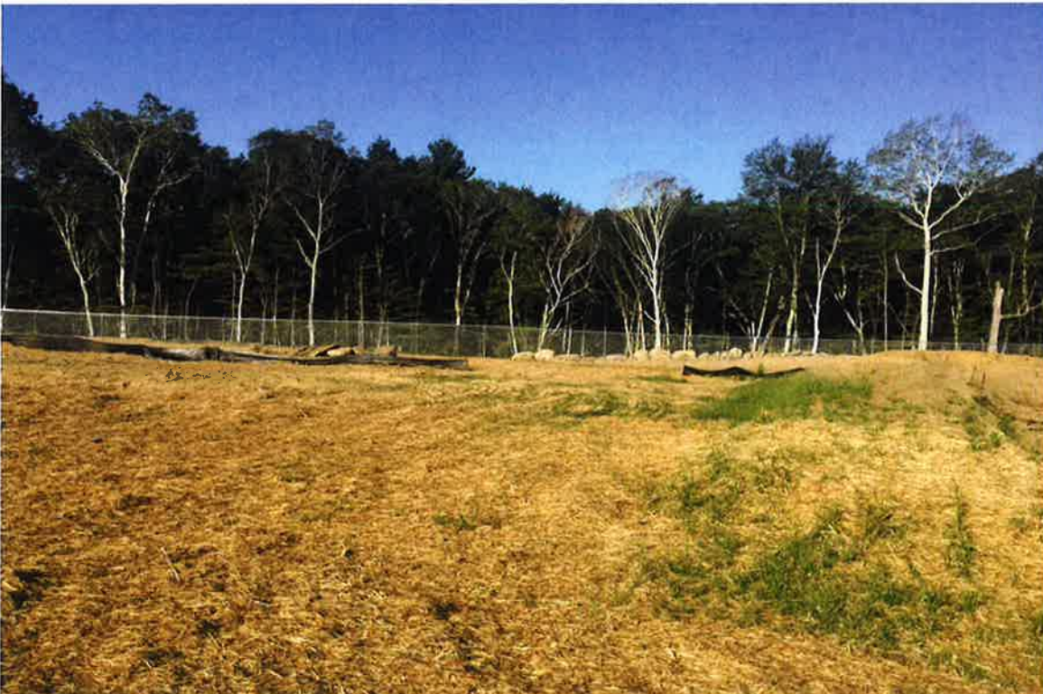
Photo 10: View of silt fence gap to be repaired.
